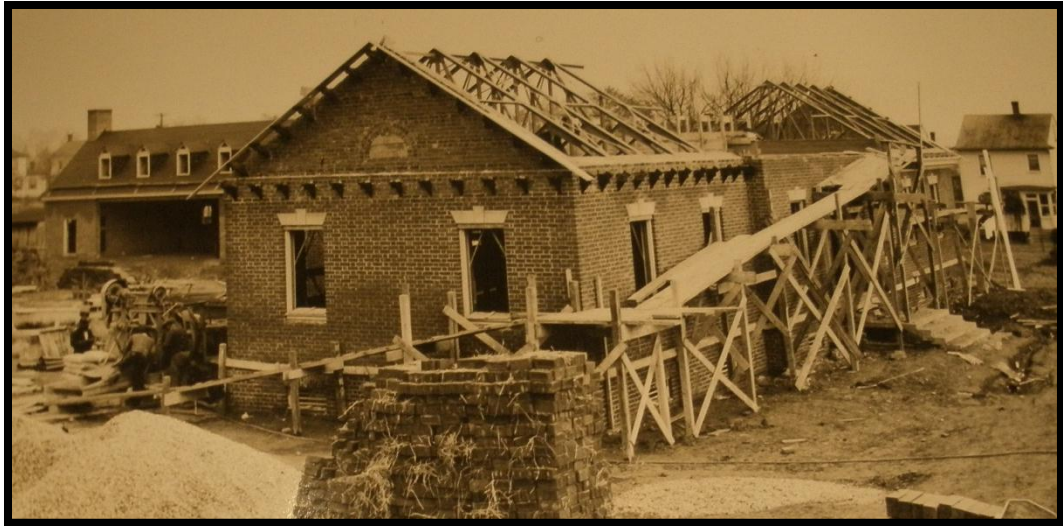
(Figure 4.18) Status of Visitor Center construction, November 1936. Courtesy of the National Archives.
