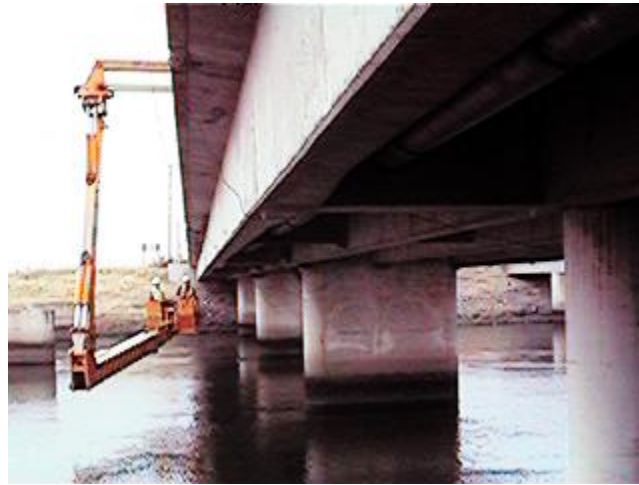
Figure 1.2: Close-up of Installation on the Byron Road Bridge in Tracy, CA.
