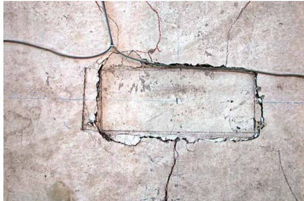
Figure 8.25: Example of Punch Failure on a Concrete Bridge Deck
