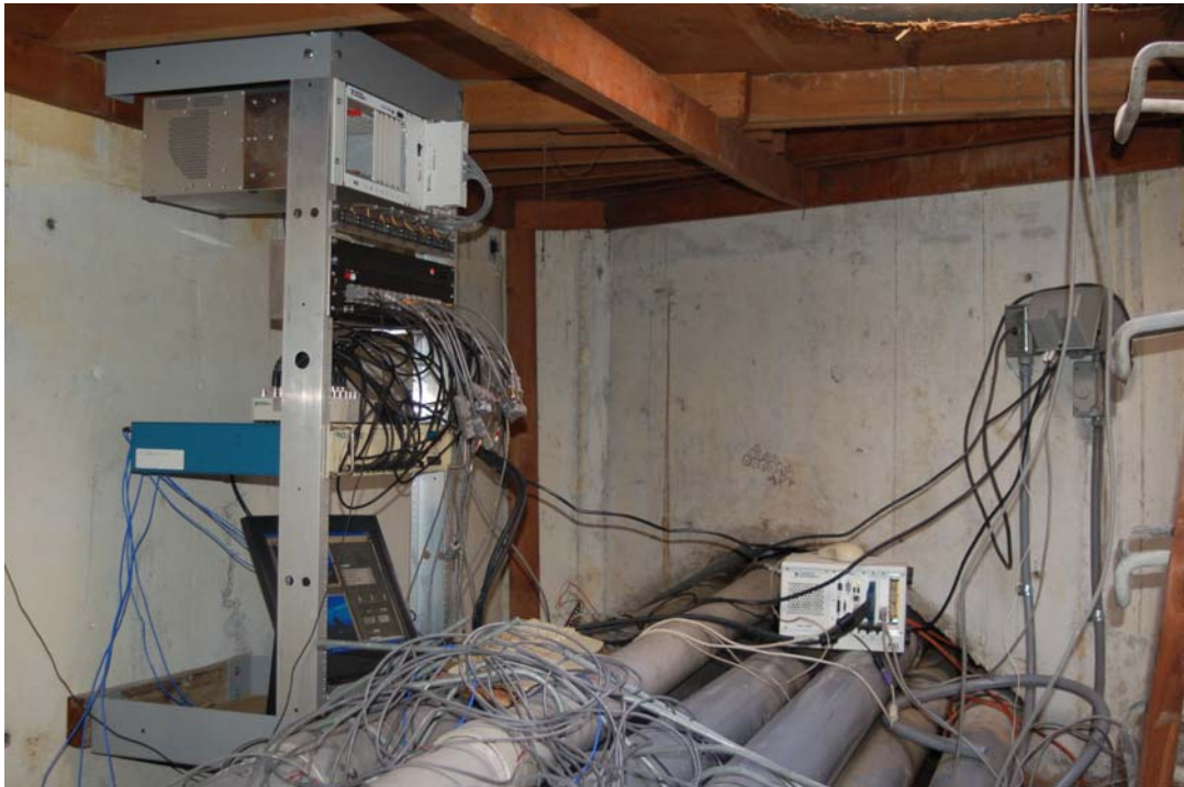
Figure 9.18: Data/Image Acquisition Hardware Installed within Bridge.
