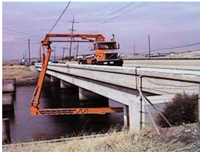
Figure 1.1: Installation of Accelerometers on the Byron Road Bridge in Tracy, CA.
