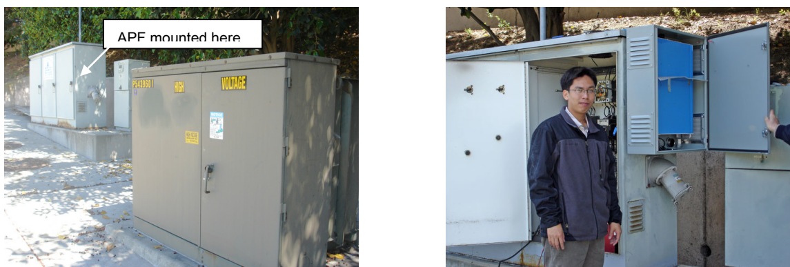
Figure 4: SMWD Site showing mounting location (left) and installed OCC-APF (right)
