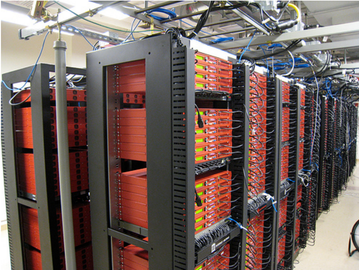
Figure 1: The “red boxes” that used to form the Archive’s machine cluster. This photograph was taken in its former data center in downtown San Francisco. Photograph courtesy of the Internet Archive.
