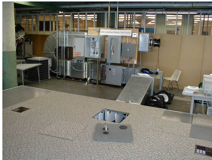
Figure 22. Photo of underfloor air supply plenum test facility
