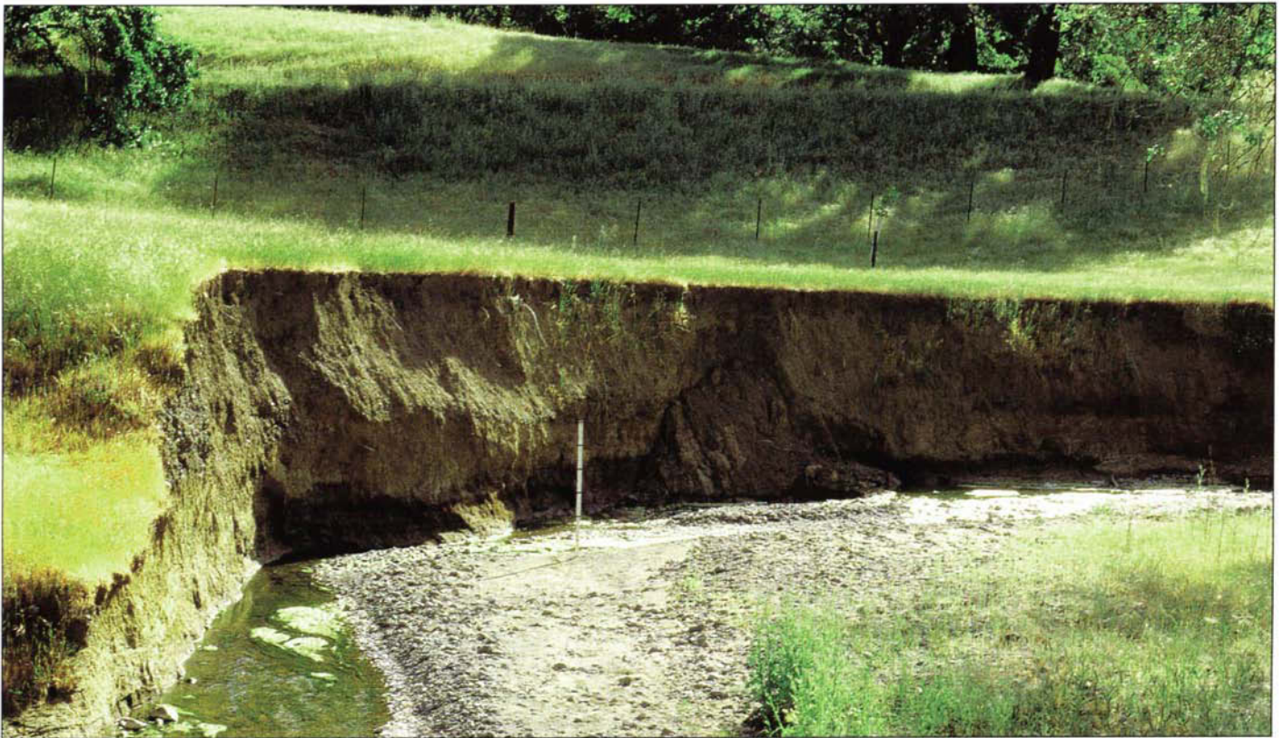
Source site of sediment delivery associated with gully erosion and resulting from road drainage management and culvert design. Current water-quality regulations require inventory, monitoring and mitigation of this site.
