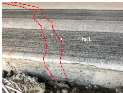
Figure 13. A zoomed-in view of B4 after 11,000 cycles of loading. The observed crack location is highlighted in red.
