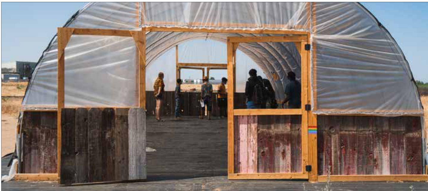
Hoop house at the Yosemite Village Permaculture Community Garden & Urban Farm Incubator, which was constructed in March 2021 and will be used as a nursery production site. Photo credit: Chris De León
