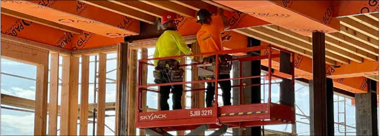
Construction of The Monarch @ Chinatown, a TCC-funded affordable housing development. Photo credit: Fresno Housing
