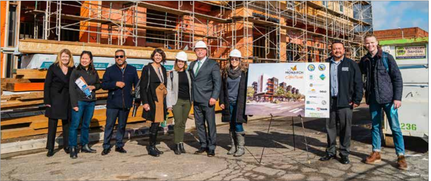
State partners on a site visit at The Monarch construction site in December 2021. Photo credit: California Strategic Growth Council
