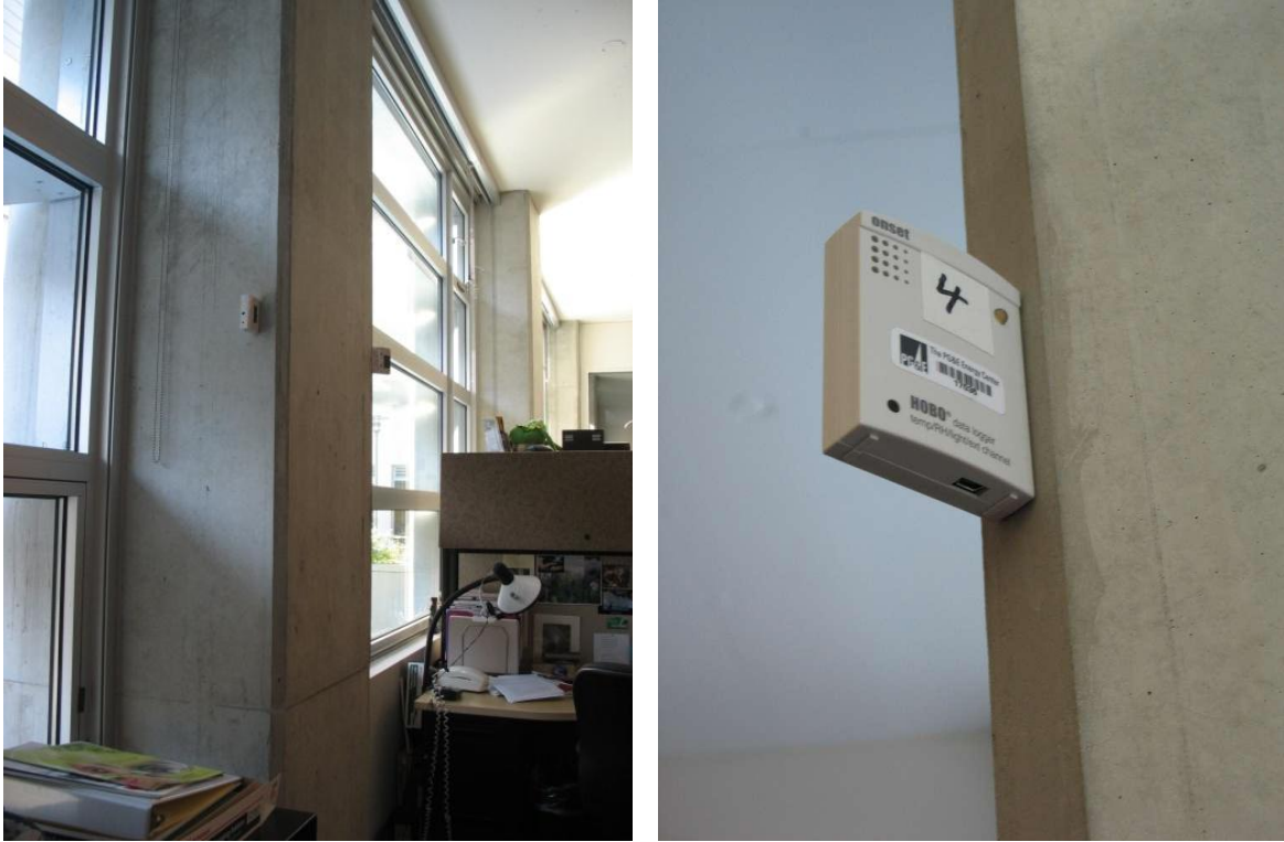
Figure 39 HOBO RH/Temp/Light data loggers used for monitoring shade deployment
