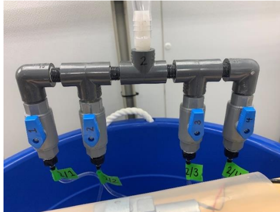
A9 The assembled and labeled 4-way valve unit. Close-up of assembled 4-way valve unit with blue 4-way valves and tubing leading from 4-way valve unit to clearly labeled cores.
