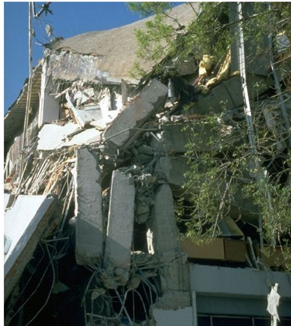
Figure 2.1(b) Structure collapse due to failure of deficient beam-column joints, Moehle [96]
