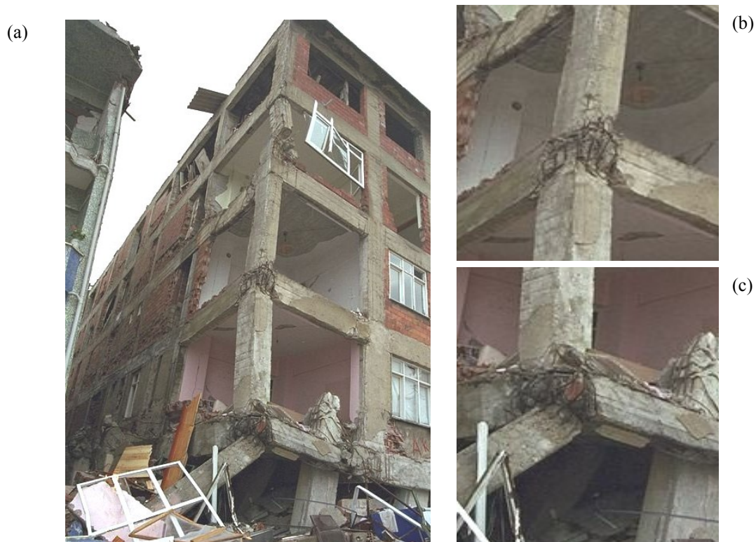
Figure 2.2 (a) Partial Building Collapse due to failure of beam-column joints in the Izmit, Turkey earthquake of August 17, 1999, (b) close-up of third-level joint, (c) close-up of second-level joint, (Courtesy of NISEE, University of California, Berkeley [106])
