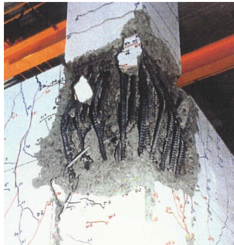
Figure 3.22 Axial failure mode of "As Built" corner joint, Priestley and Hart [129]
