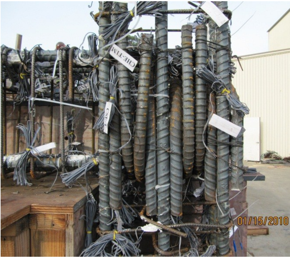
Figure 6.7 Congested beam reinforcement steel hooks inside the joint
