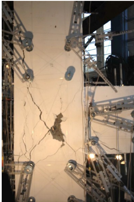
Figure 7.152 Torsional cracking of EW beam during NS beam downward loading in specimen U-J-1
