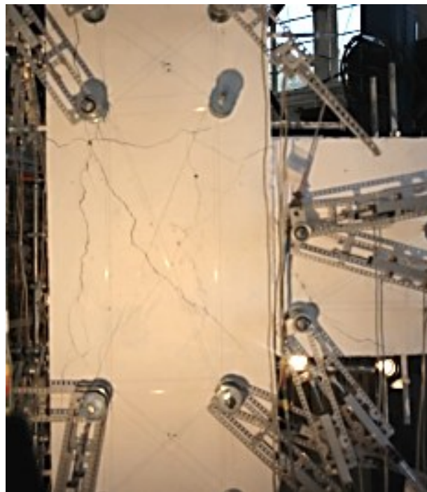
Figure 7.4 Characteristic joint panel cracks
