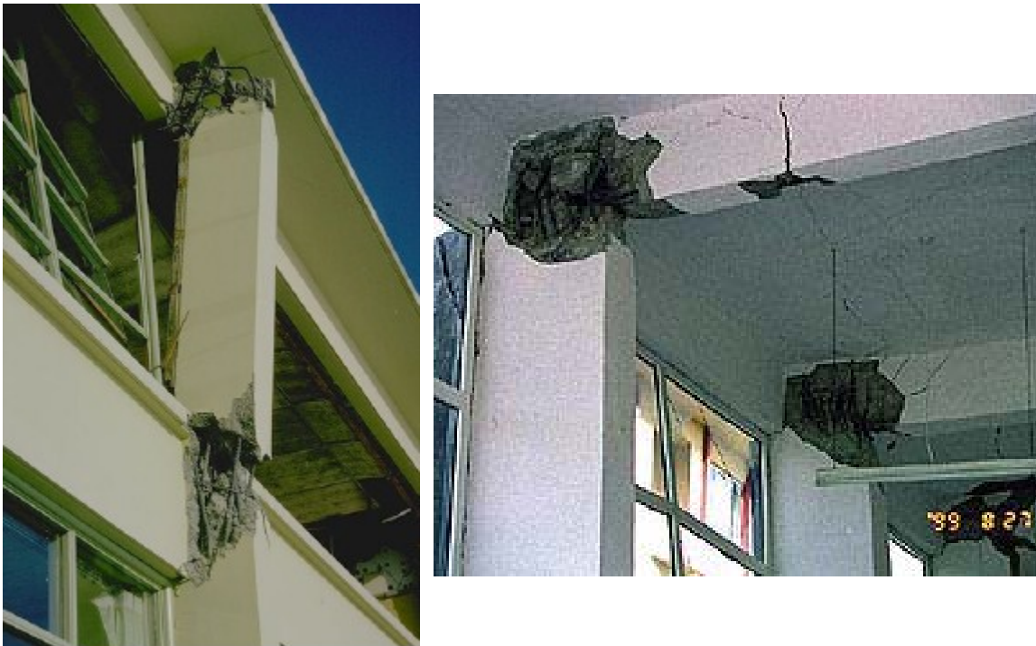
Figure 2.8 Severe exterior joint earthquake damage, Lehman [82]
