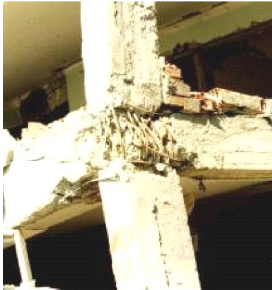
Figure 2.5 Corner beam-column joint damage in the Izmit, Turkey, earthquake of August 17, 1999, photo credit: Güney Özcebe, Engindeniz [41]
