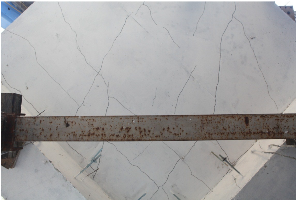
Figure 7.157 Crack pattern of slab in specimen B-J-1
