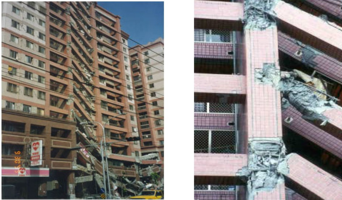
Figure 2.3 Damage to partially collapsed 15-story building: beam-column failure in Chi-Chi, Taiwan, earthquake of Sep. 21, 1999, Uang et al. [149]
