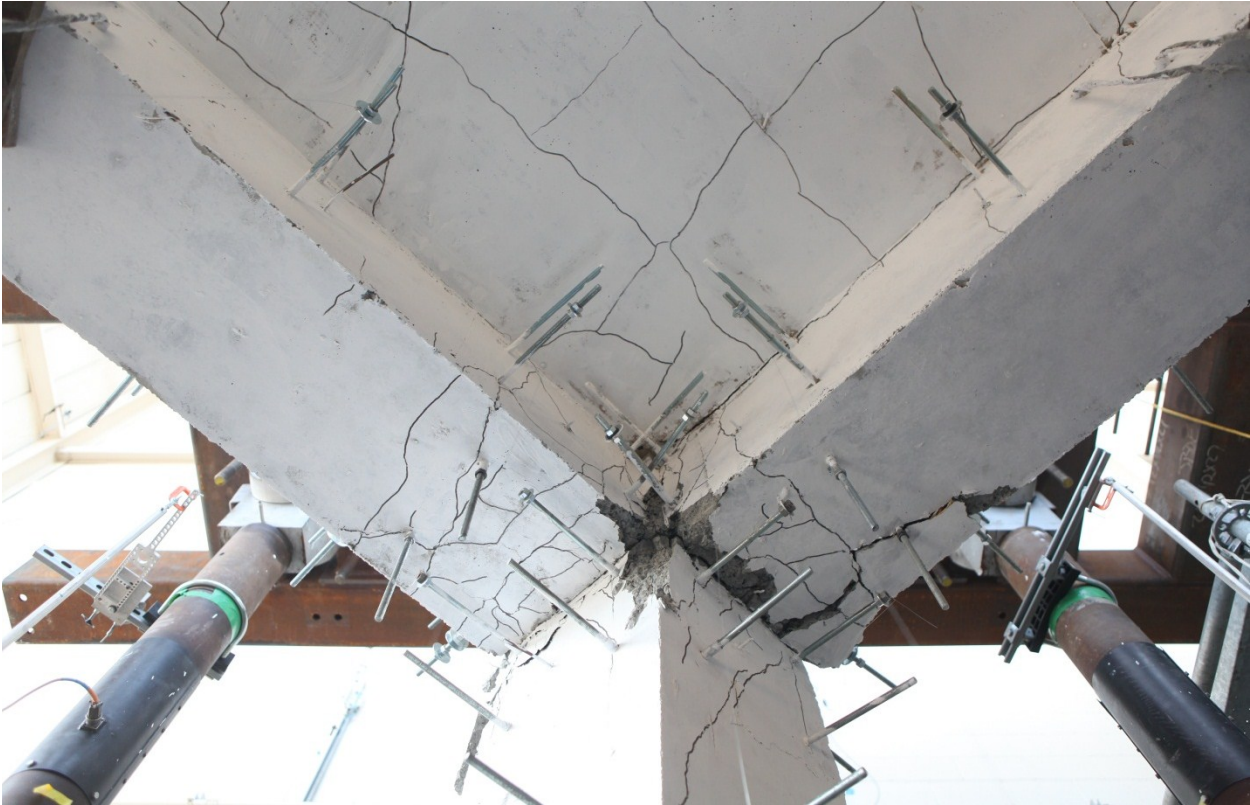
Figure 7.141 Crack pattern of slab in specimen U-BJ-1
