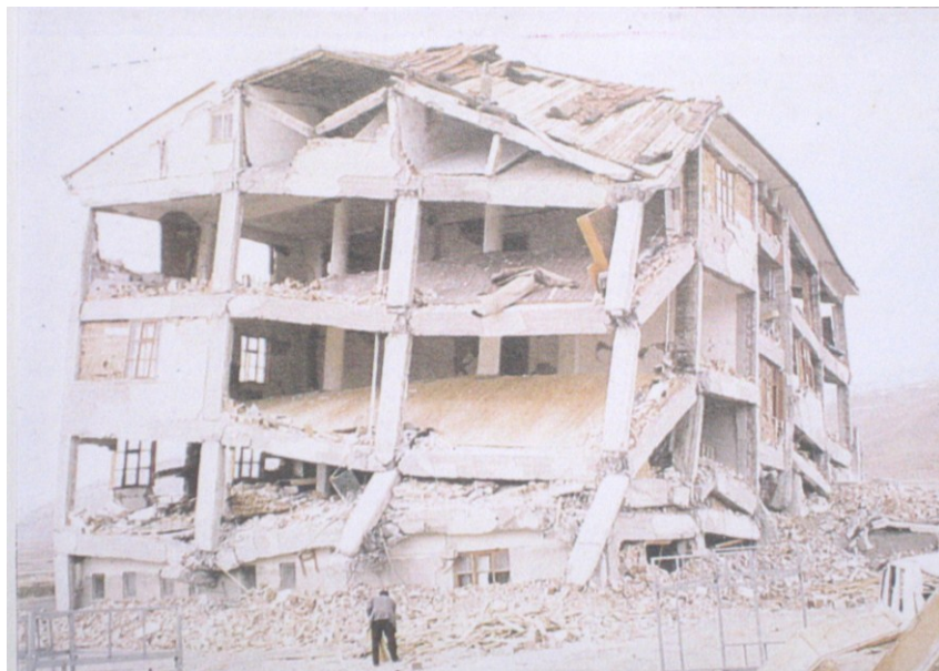
Figure 2.6 Joint failure and partial building collapse in the March 13, 1992, Erzincan, Turkey earthquake, Zahertar [158]
