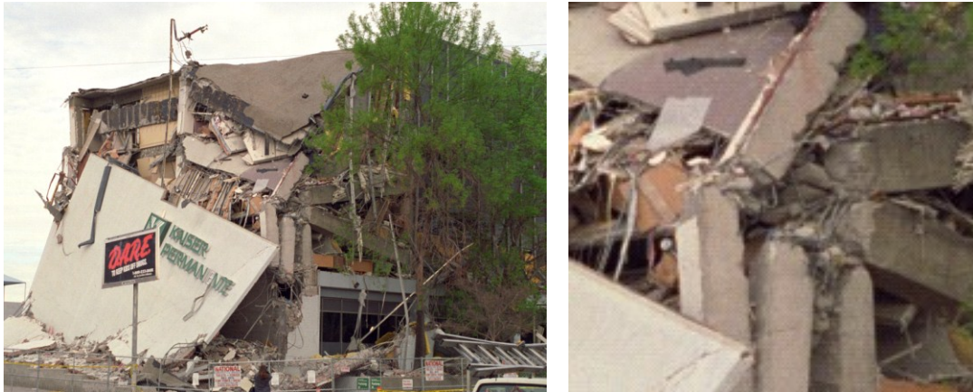
Figure 2.1(a) Structure collapse due to failure of deficient beam-column joints, Kaiser Permanente Building, Northridge earthquake, 1994 (photo credit, G. Edstrom)
