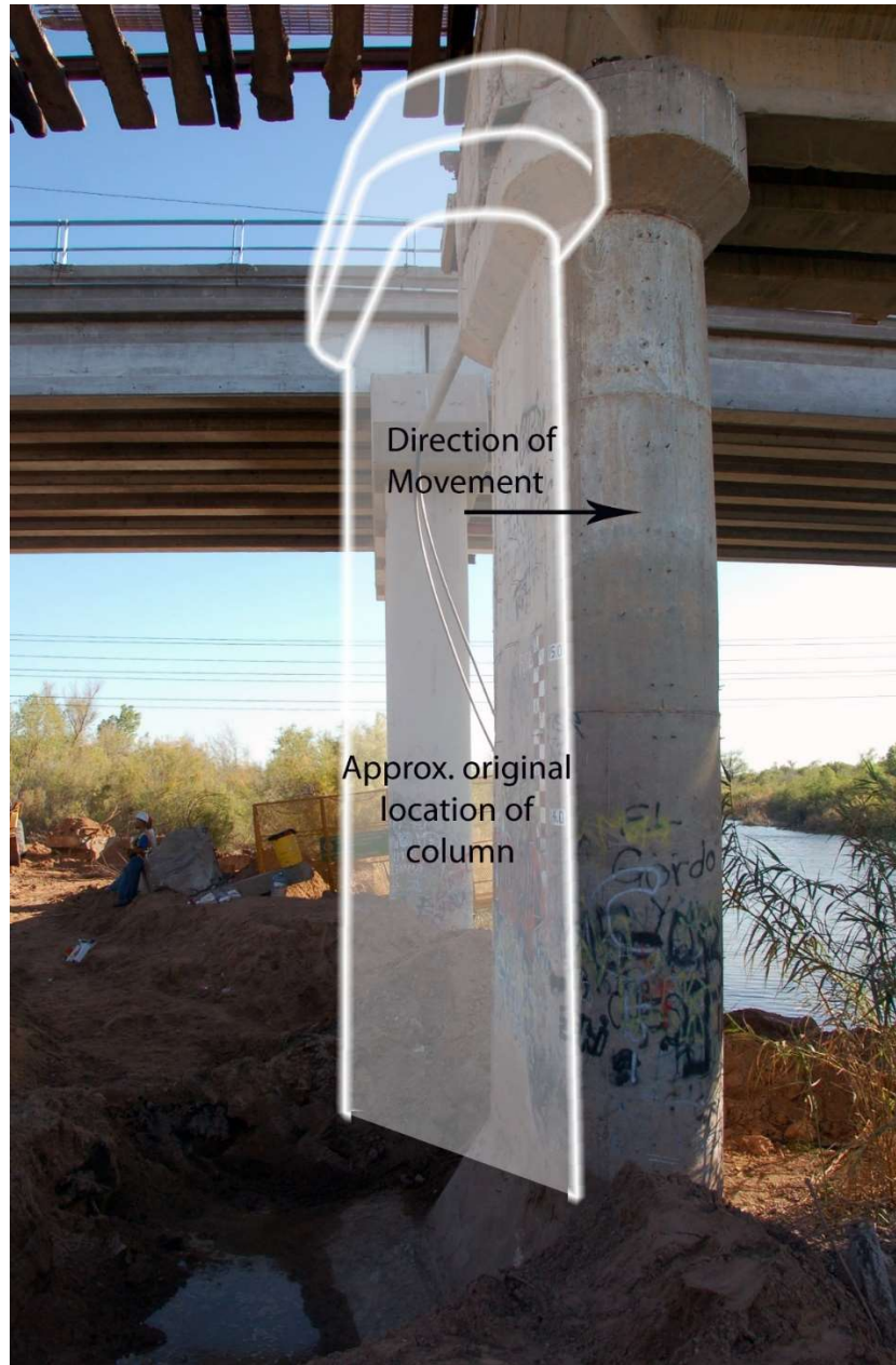
160 161 Figure 3: Bent 5 of railroad bridge (foreground) that translated towards river causing 162 unseating collapse, and Bent 5 of highway bridge (background) following 2010 El Mayor- 163 Cucapah earthquake. Photo J. Gingery/GEER (2010).
