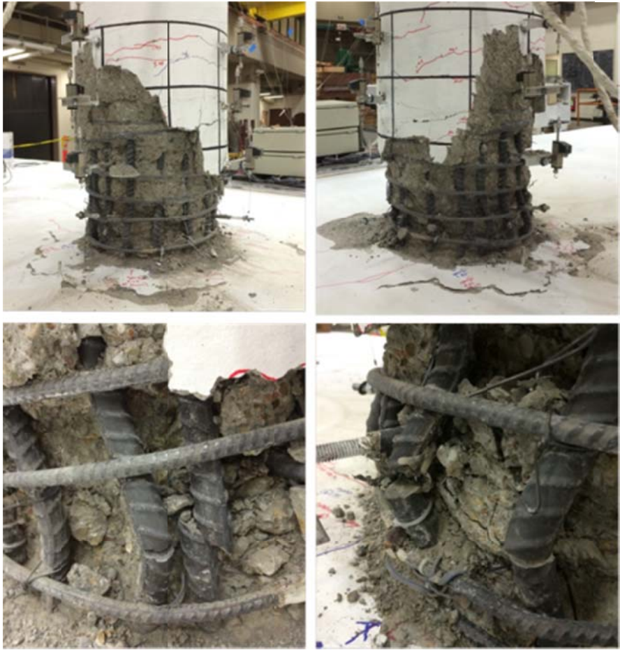
Figure 5.6 Final damaged state of the as-built SP1 column: all the rebars were exposed and buckled, and six rebars were ruptured
