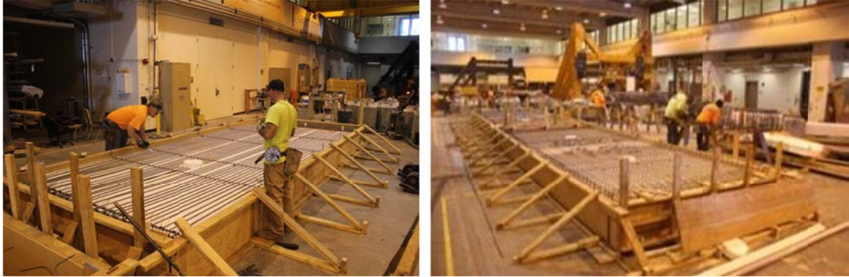
Figure C.3 laying out the deck slab longitudinal and transverse reinforcement and installing two styrofoam cylinders to construct the 9-inch holes for actuator rods to pass through (left); final completed deck slab reinforcement mesh (right)
