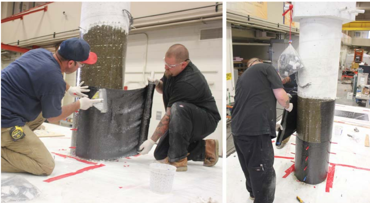
Figure 8.4 Applying the first CFRP layer of the lower part of the jacket (left) and of the upper part of the jacket (right) of the column using the ready CFRP wet rolls
