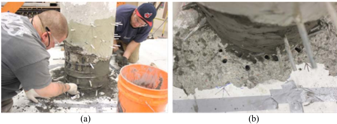
Figure 6.4 (a) Patching the column damaged core with high-strength mortar in the plastic hinge zone; (b) 8-inch deep vertical holes to add polymer reinforcing bars
