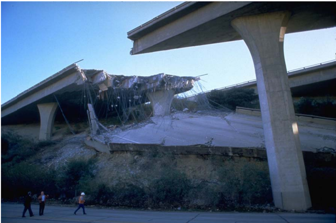
Figure 1.3 Damaged portion of the Golden State Freeway, part of CA Interstate-5, at Gavin Canyon after 1994 Northridge earthquake (courtesy of FEMA Photo Library)
