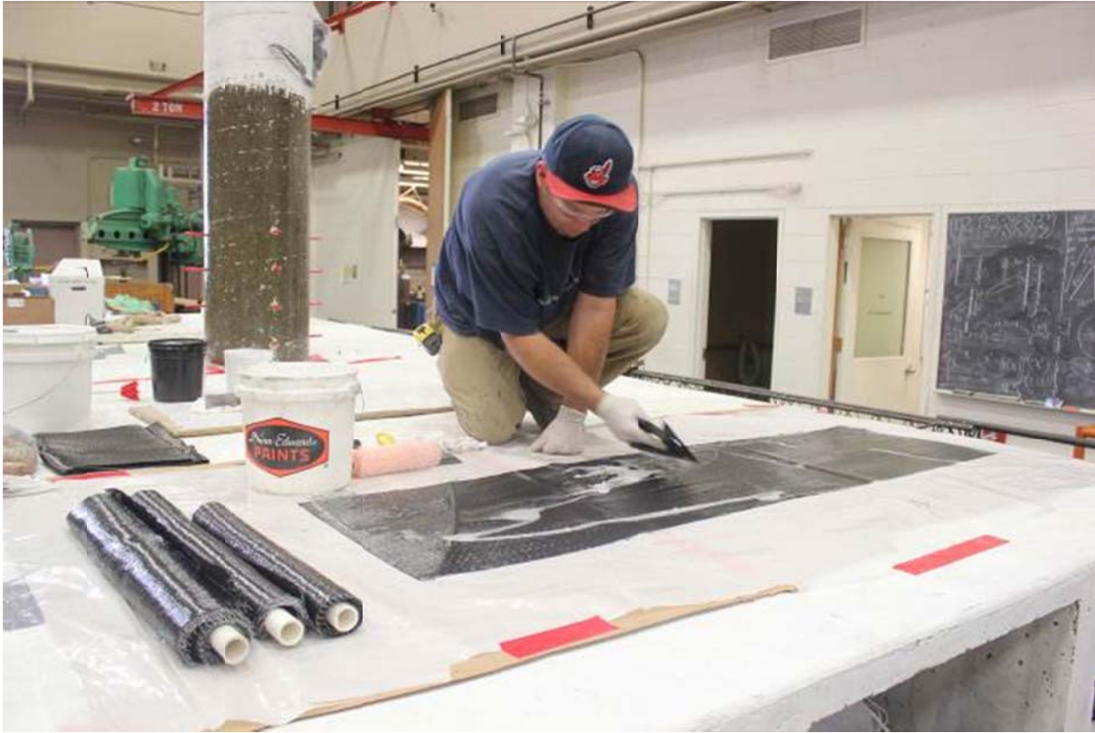
Figure 8.3 Coating the carbon sheets with epoxy resin and rolling the wet sheets in preparation for wrapping
