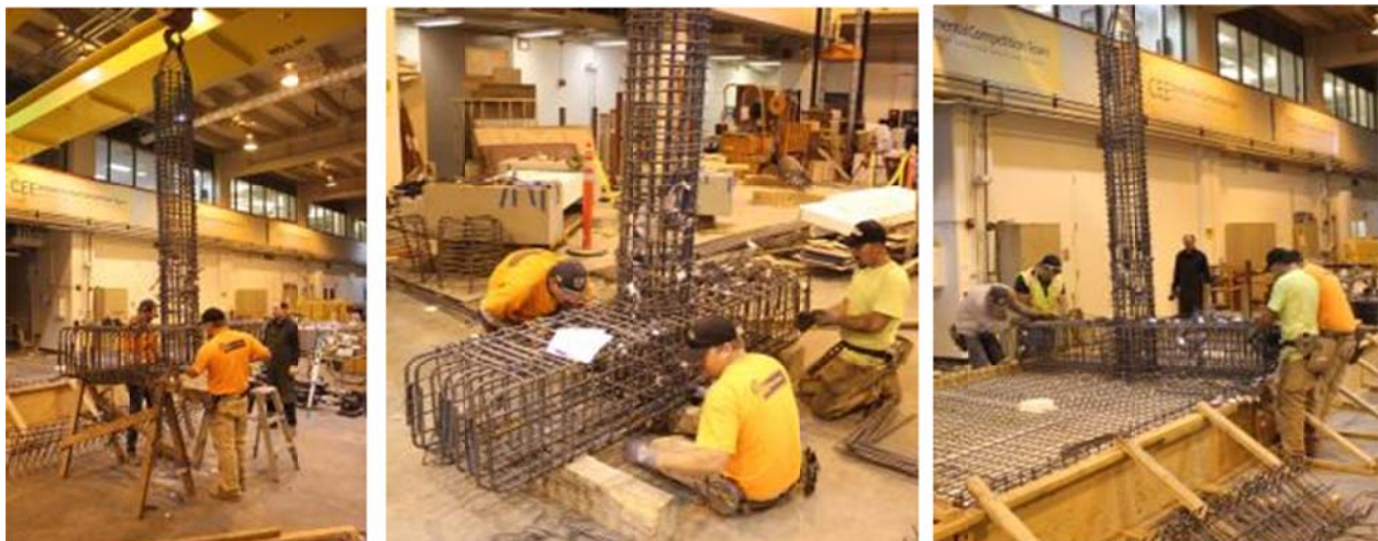
Figure C.5 Different stages of assembling the bent cap beam and column cages then installing the assembly in place using the overhead crane
