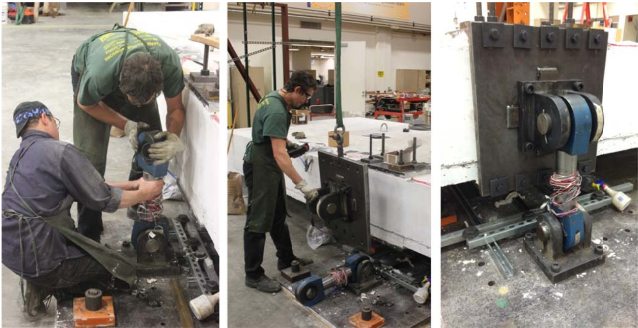
Figure D.8 Assembling one of the vertical struts using the instrumented load cell and two clevises (left); aligning and attaching the side plate used as part of the vertical strut connection (middle); final vertical strut connection at one of the bent cap beam ends
