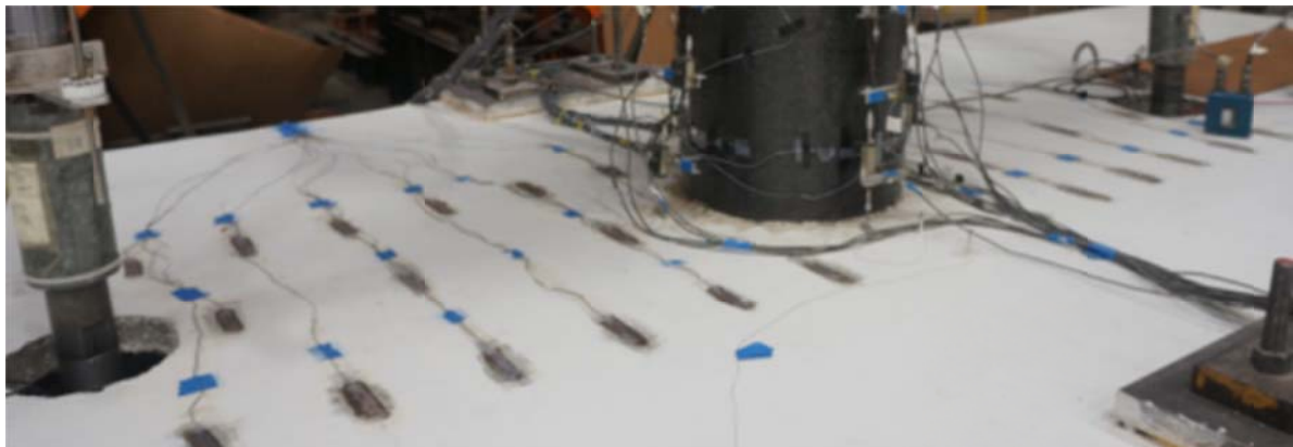
Figure 3.44 Surface concrete strain gages installed on top of the soffit slab of the second specimen only (some CFRP jacket strain gages are shown also)
