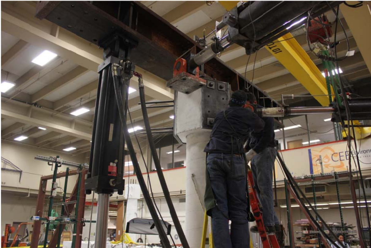
Figure D.12 Attaching the two horizontal actuators to the column head to complete the last step of the test setup procedure
