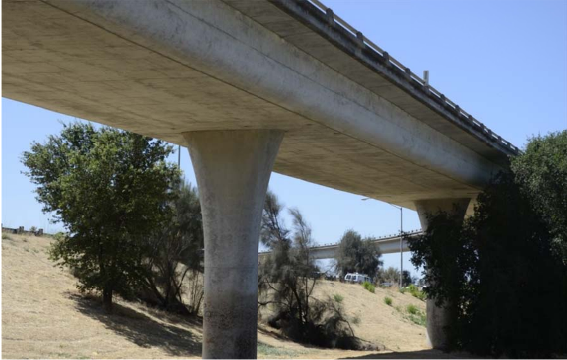
Figure 1.2 Typical California box-girder bridge: W80-E50 Connector Overcrossing, Yolo County, California (courtesy of Mark Yashinsky, Caltrans)
