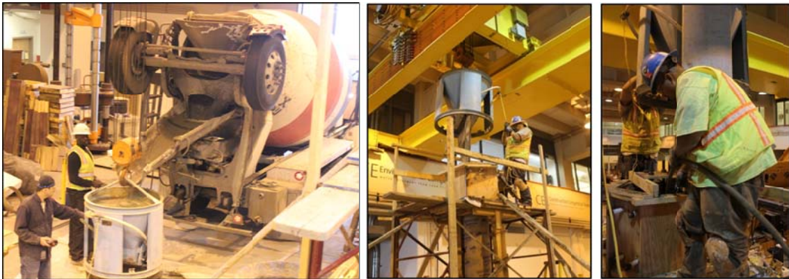
Figure C.13 Placing concrete into an overhead hopper for the concrete third lift (left); moving the hopper using the overhead crane (middle); and placing and vibrating the concrete of the column and column head (right)
