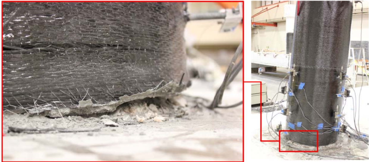
Figure 6.14 Circumferential tear in the CFRP jacket and cracking at the column-bent cap interface as lateral loading progressed
