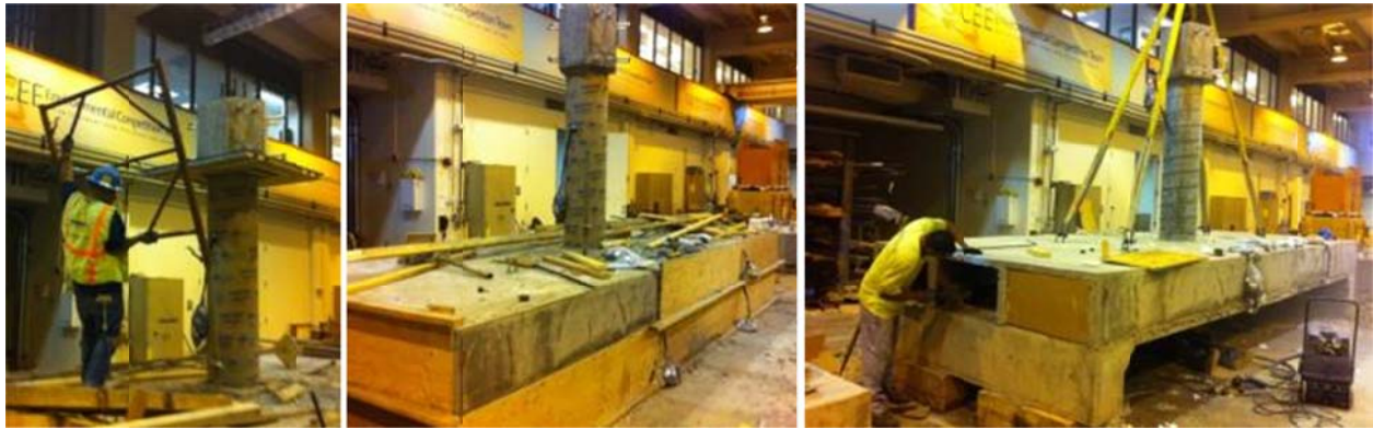
Figure C.15 Removal of column scaffolding (left), side formwork (middle), and inside cardboard boxes (right)
