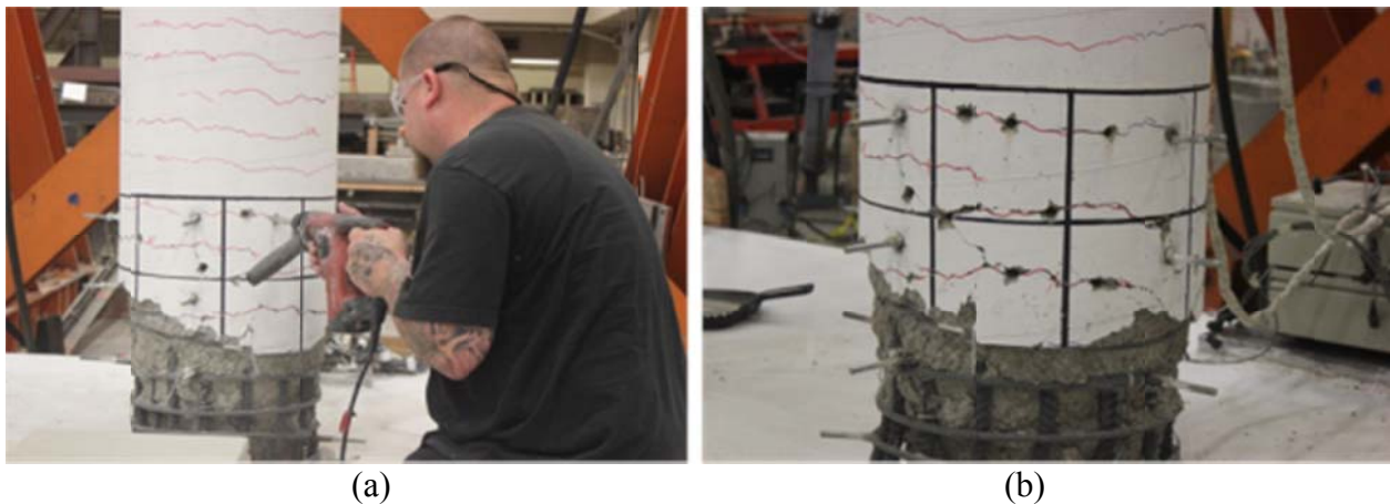
Figure 6.2 (a) Drilling holes along the cracks for epoxy injection; (b) final holes pattern for cracks injection
