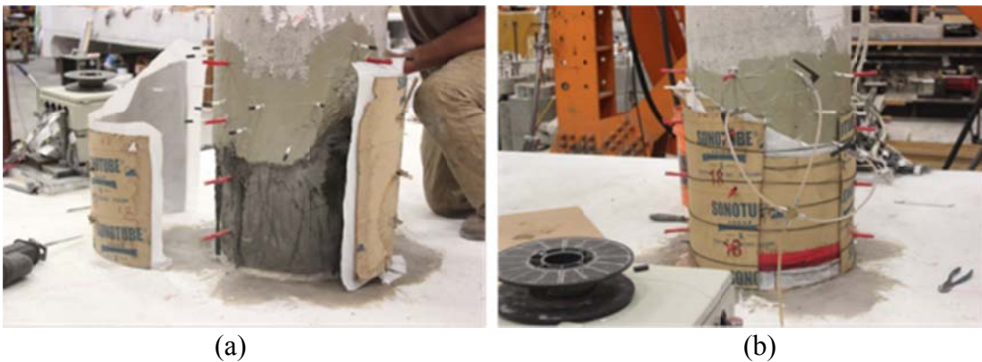
Figure 6.7 (a) Installing sonotube around the damaged zone to restore the column's circular shape; (b) injecting fluid epoxy into the cracks using the installed injection ports
