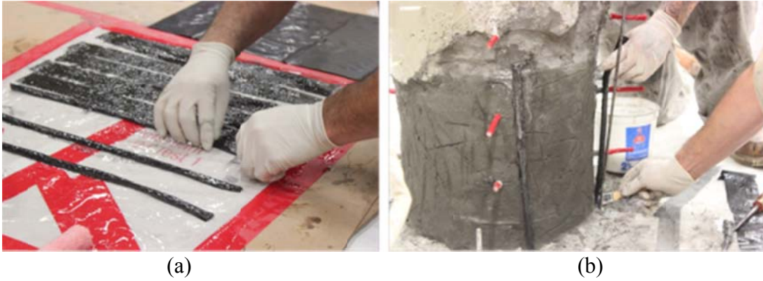
Figure 6.5 (a) Preparation of 20-inch long CFRP bars using carbon fiber sheets coated with epoxy resin; (b) installing the wet CFRP bars in the holes drilled into the cap beam
