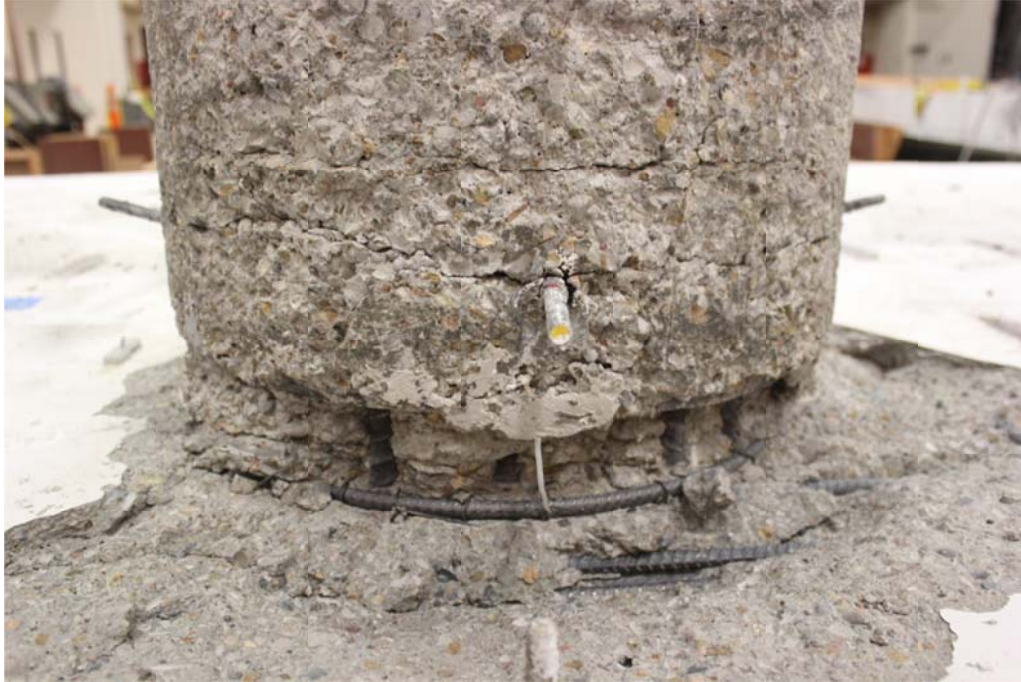
Figure 8.9 A close-up view of SP2 column flexural cracks (CFRP jacket was removed) and bent cap beam concrete cover spalling after HS tests
