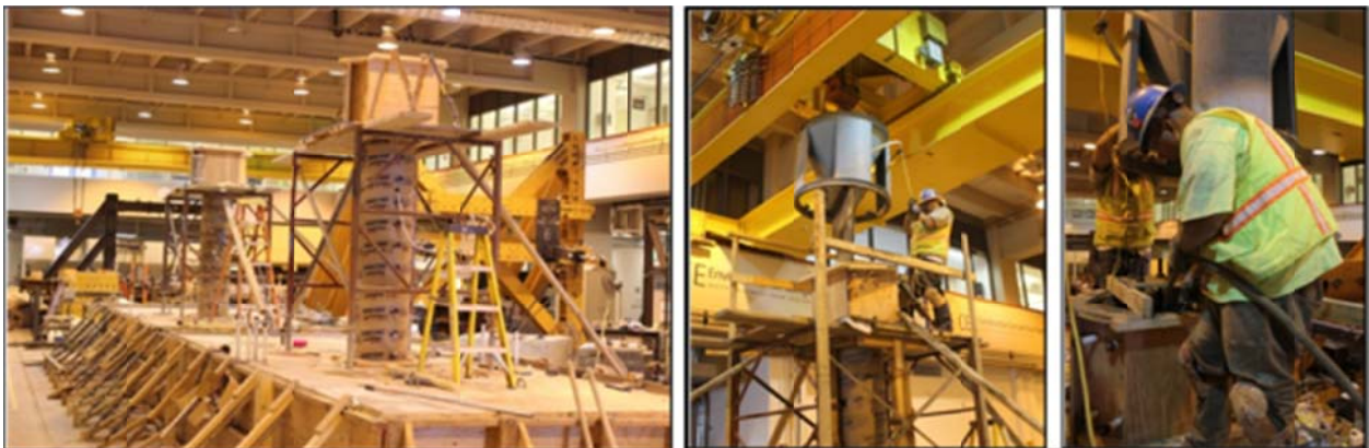
Figure 3.21 Column and column head formwork (left) and placing and vibrating the concrete of the column and column head (middle and right)
