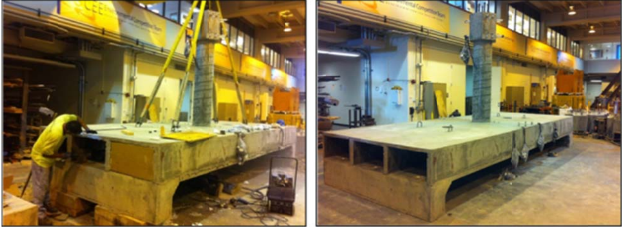
Figure 3.22 Removing the cardboard boxes used to create the box-girder cells (left) and final specimen configuration (right)
