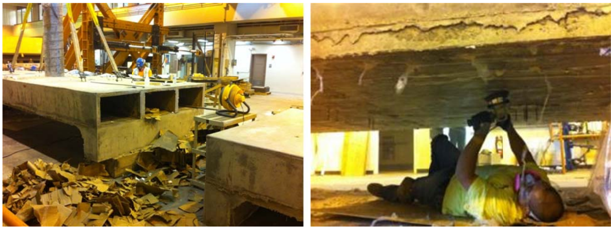
Figure C.16 Ripping all the cardboard boxes from inside the box-girder cells (left); and grinding any styrofoam or plastic wrap stuck to the concrete surface (right)
