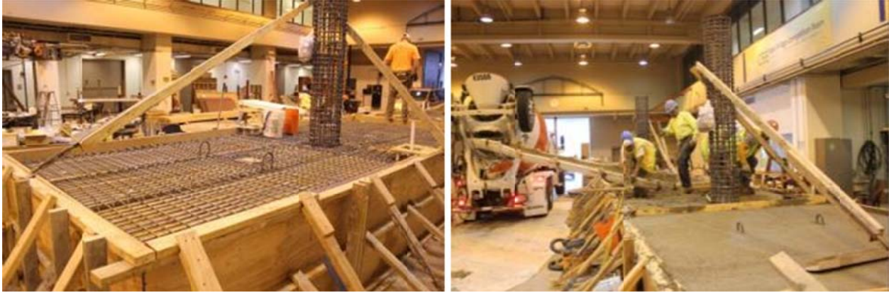
Figure C.9 Laying out the soffit slab reinforcement mesh (left); and casting the box-girder soffit slab and cap beam concrete second lift (right)
