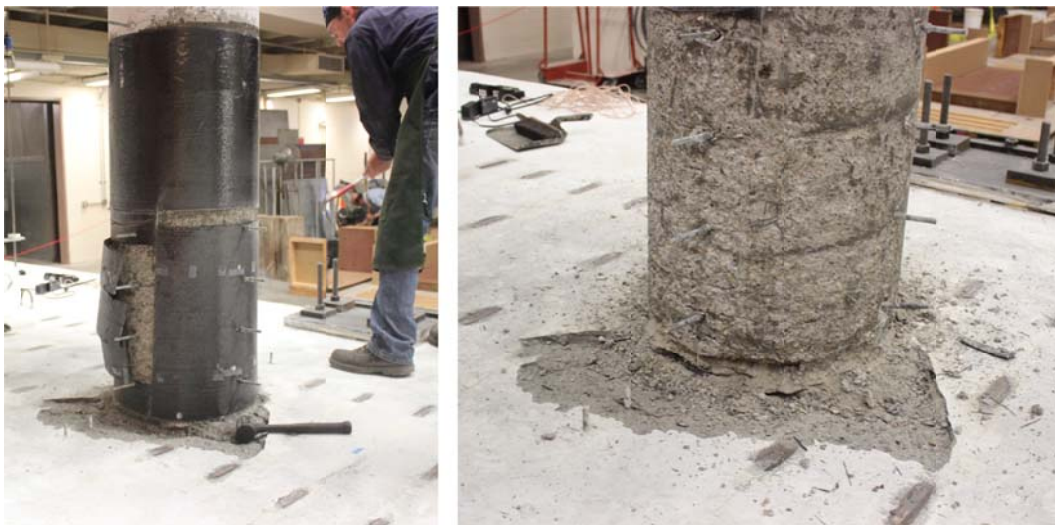
Figure 8.8 Procedure of removing the CFRP jacket after the retrofitted SP2 tests were concluded (left) and final view of the column after the jacket removal (right)
