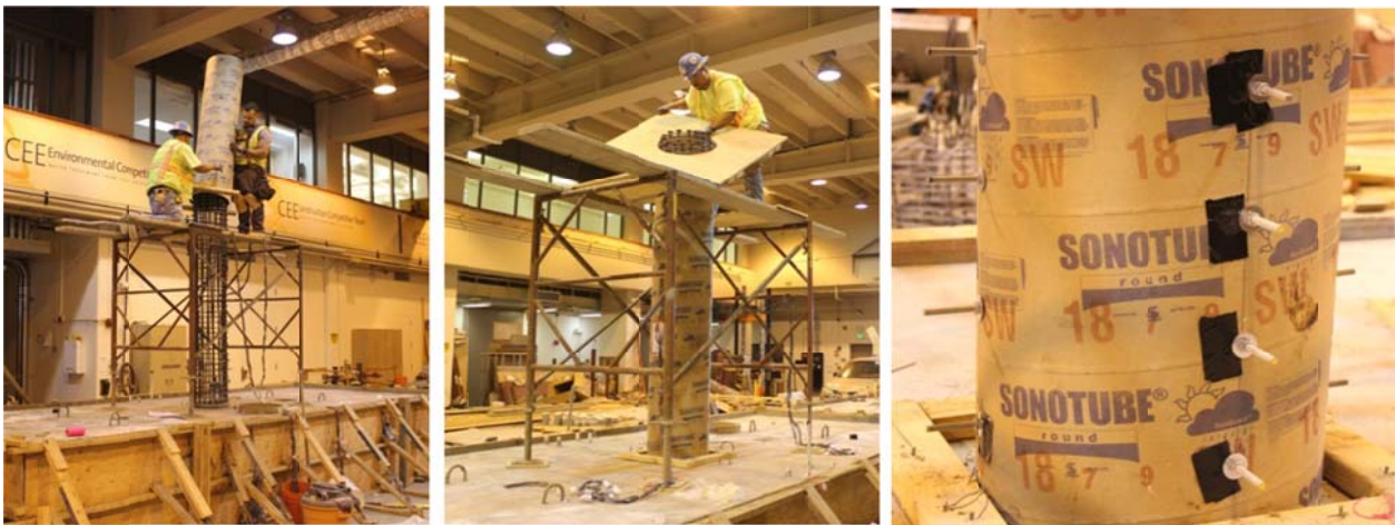
Figure C.11 Installing the column sonotube (left); building the column head scaffolding (middle); and inserting instrumentation rods into the column formwork (right)
