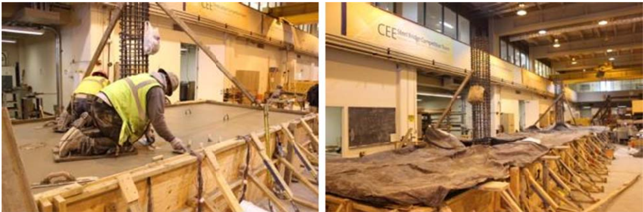
Figure C.10 Finishing the surface of the second concrete lift (left); and using curing blankets in addition to the E-CURE to avoid any shrinkage cracks in the soffit slab (right)
