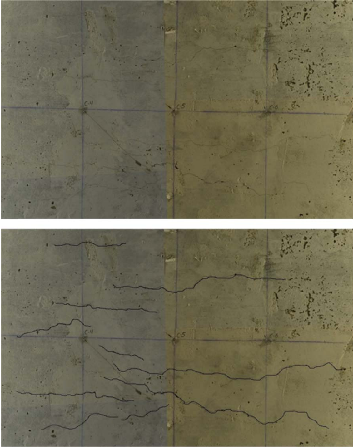
Figure 5.4 Minor flexural longitudinal cracks in the deck slab, i.e. bottom face of the inverted specimen, after all loading cycles. The horizontal line in the figure coincides with the box-girder center line
