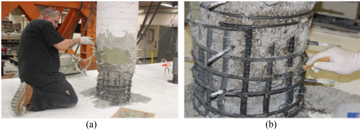
Figure 6.3 (a) Installing the injection ports along the cracks and patching the concrete surface around the ports; (b) exposed rebars coated with epoxy primer for better bond
