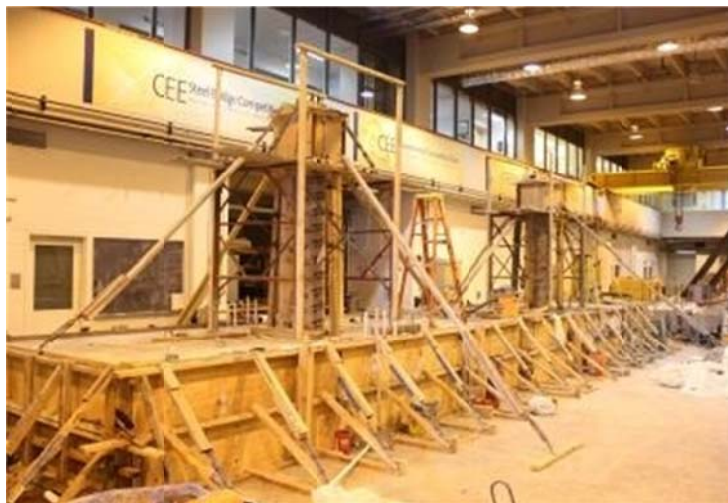
Figure C.14 The two specimens' construction after it was completed in 3 stages and left to cure for 21 days before removing the formwork
