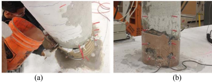
Figure 6.8 (a) Pouring sand-epoxy mixture inside the sonotube formwork to restore the column shape; (b) view of the partially repaired column after the sonotube was removed
