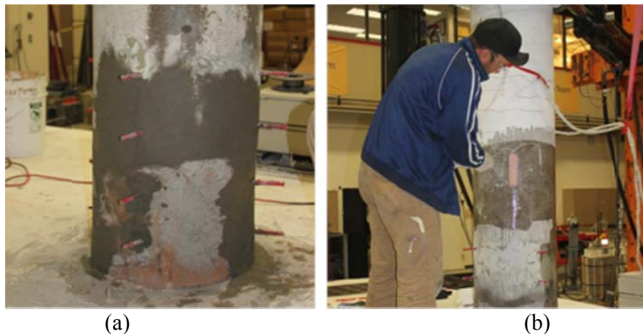
Figure 6.9 (a) A final layer of high strength mortar was applied to patch any remaining voids; (b) applying a primer epoxy coat to the surface before applying the CFRP sheets
