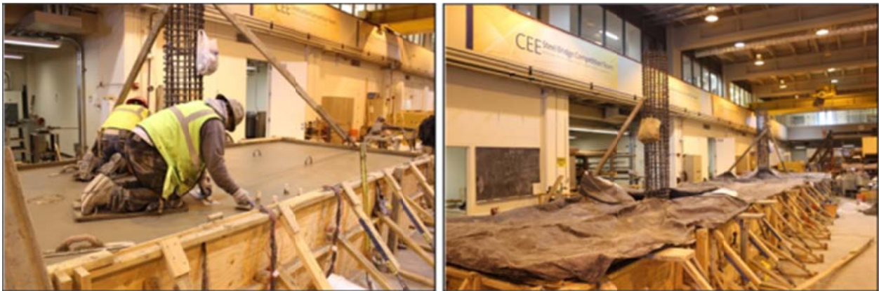
Figure 3.20 Finishing the surface of the second concrete lift (left) and curing of concrete surface using curing blankets (right)
