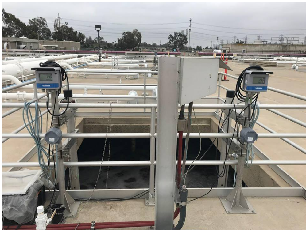
Figure 2.2: Photograph of the installation of two ammonium probes at the beginning of the aeration tank (high range conditions).
