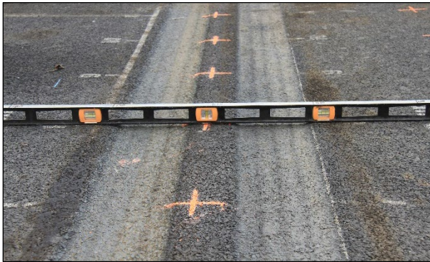
Figure 5.19: 704HB: View of rut at Station 8.
