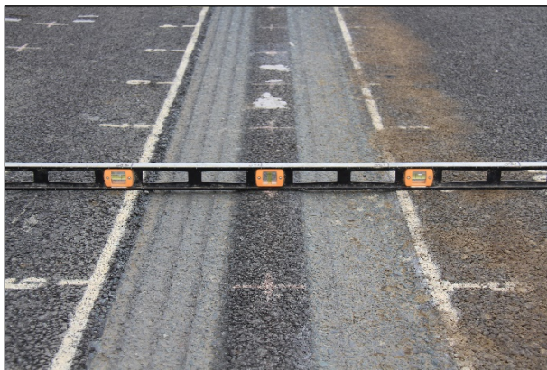
Figure 5.61: 700HB: View of rut at Station 8.
