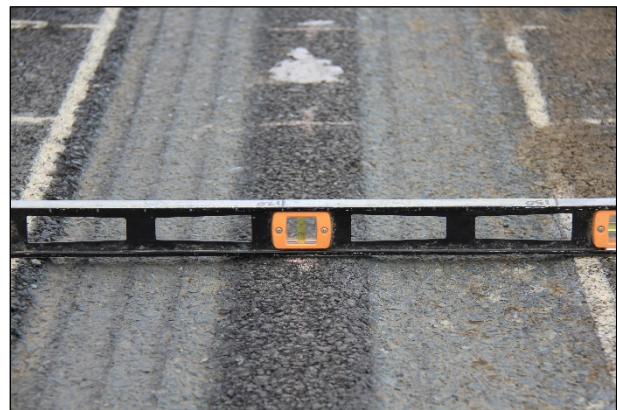
Figure 5.62: 700HB: Close-up view of test section surface at Station 8.
