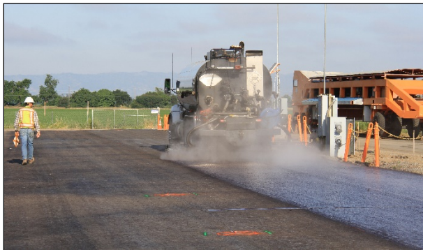
Figure 3.5: Tack coat application before first lift of RHMA-G (Sections H and I).
