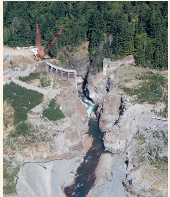
Aerial photograph of the Elwha River flowing through the remains of the Glines Canyon Dam during the third year of the dam removal project. Photo by Jeffrey Duda, USGS
