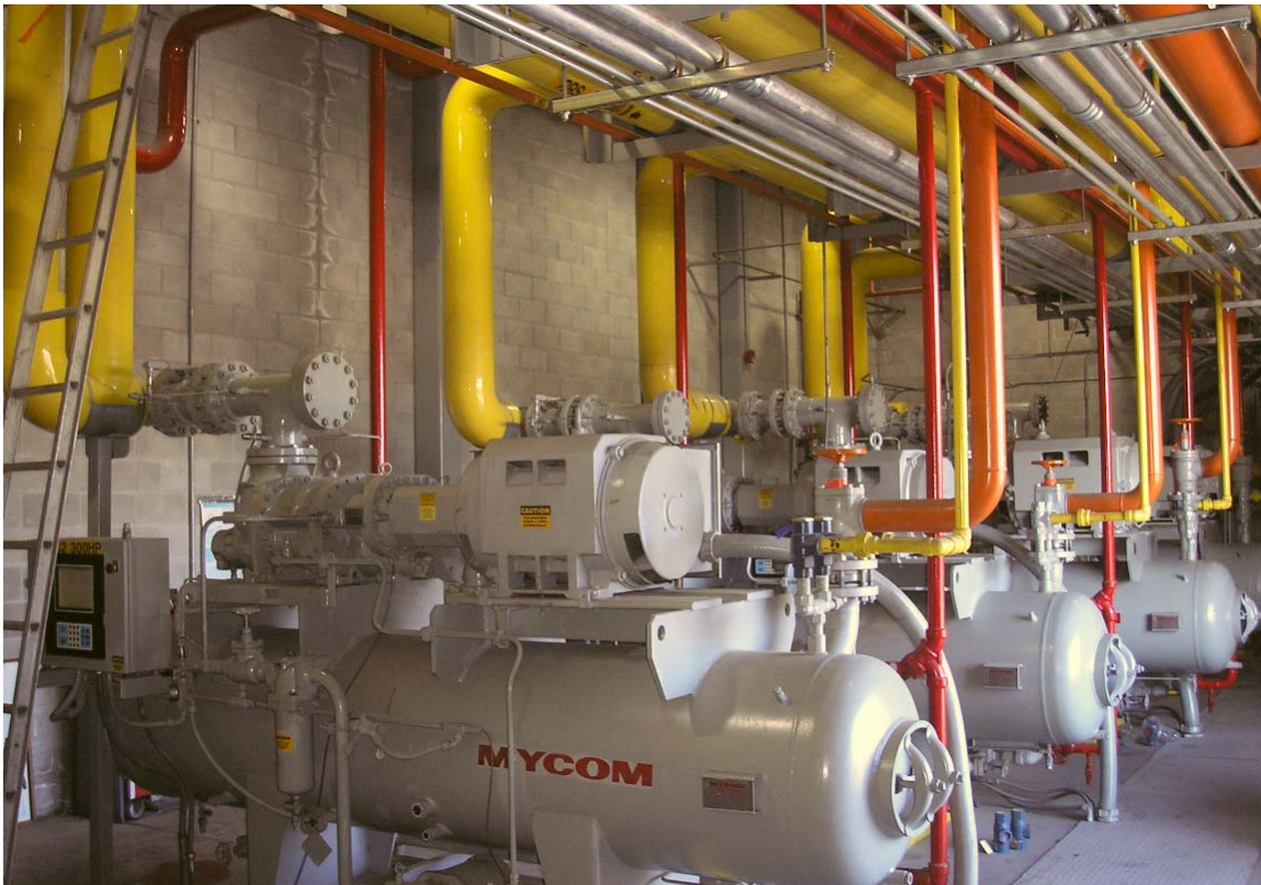
Figure 3. Example of a Custom Built-Up Refrigeration System
