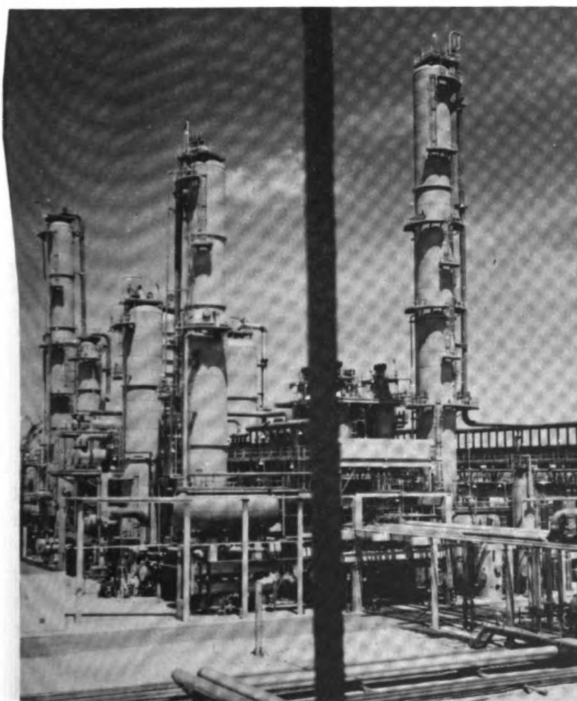
Figure 1-11 Distillation towers in the aromatics recovery unit at the Texas City, Texas, refinery of the American Oil Company. ( Pullman Kellogg Co. )
