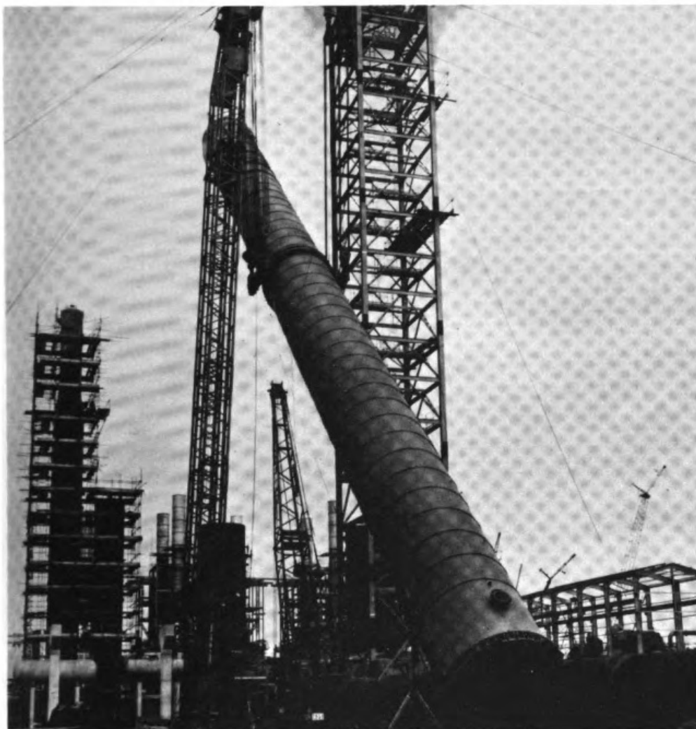
Figure 4-7 A giant distillation column, 82 m high and 4.9 m in diameter, being lifted into place at the Imperial Chemical Industries, Ltd., ethylene plant at Wilton, England. This plant produces ethylene, propylene, and butadiene from hydrocarbon feedstocks derived from petroleum refining. Note the scaffolding surrounding the towers under construction in the background. ( The Lummus Co., Bloomfield, N.J. )
