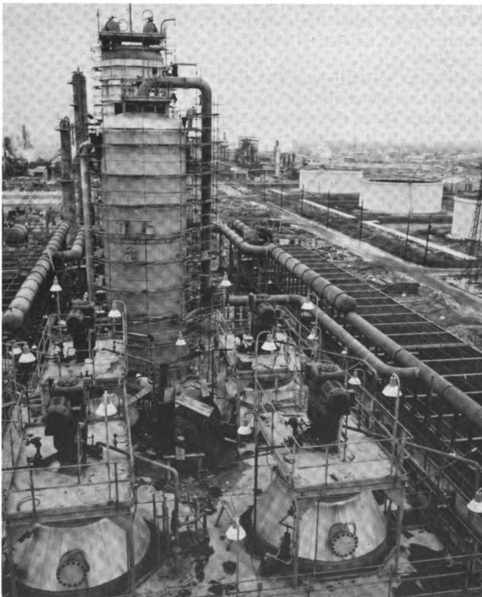
Figure 1-10 Rotating-disk contactors used for the extraction of aromatics from other hydrocarbons in the aromatics recovery unit at the Texas City, Texas, refinery of the American Oil Company. The RDC vessels are each 20 m long and 3.4 m in diameter. The solvent in this plant is Sulfolane. ( Pullman Kellogg Co. )
