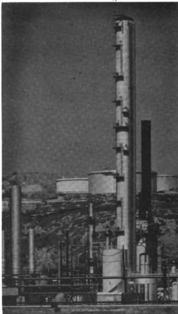
Figure 14-3 A xylene splitter column at the Richmond, California, refinery of Standard Oil Company of California. This column takes m - and p -xylenes as distillate and o -xylene as bottoms. Notice the large size compared with other columns. (Chevron Research Company, Richmond, California.)
