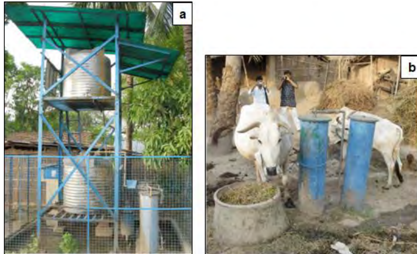
Fig. 14.1 Arsenic Removal Units (ARUs) in Murshidabad District of West Bengal, India. Panel a), a working ARU, (typical for 5% of installed units at 1-year after installation). And, Panel b), a defunct ARU, (typical of 95% of units at 1-year after installation)
