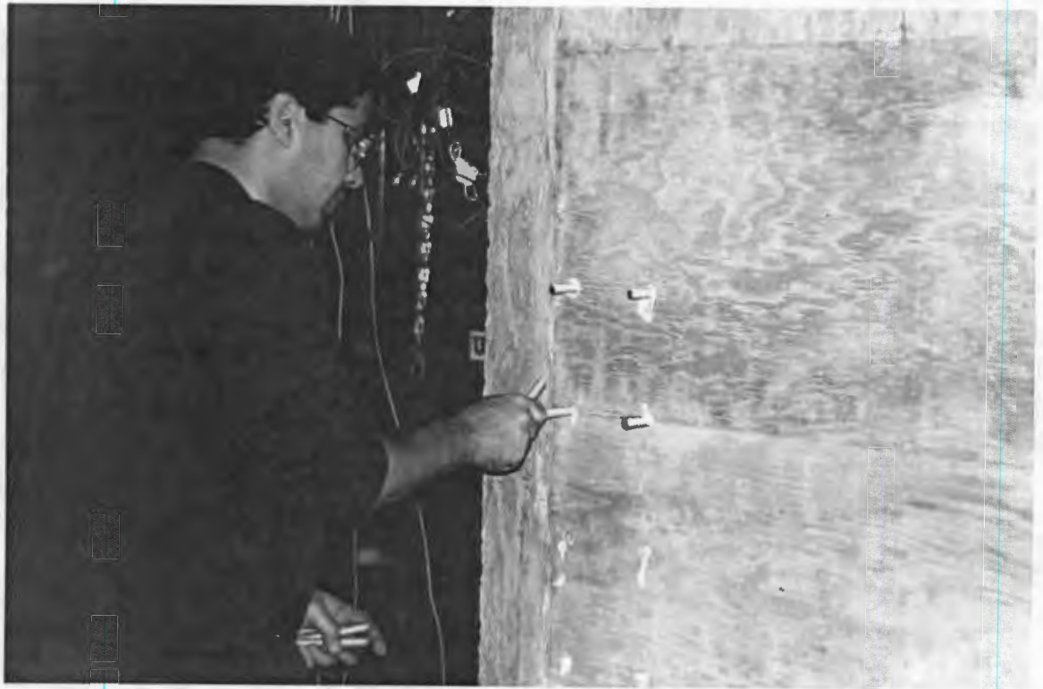
Figure 5.3. Installation of Hilti Hit HY-150 at the bottom support: (a) injection of the epoxy, (b) installation of the studs
