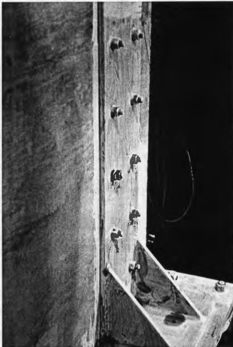
Figure 7.14. Some nuts loosened up after test no. 18
