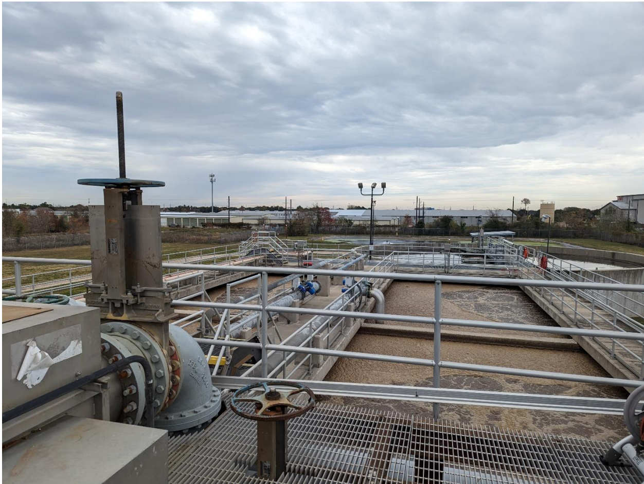
Figure 5: Water treatment plant owned by MUD 418
