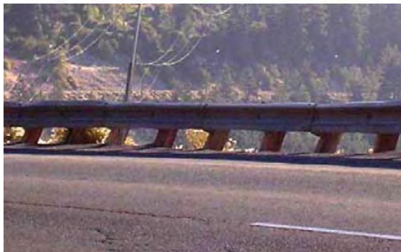
Figure 1. 1 Two sections of guardrail damaged by snowblower
