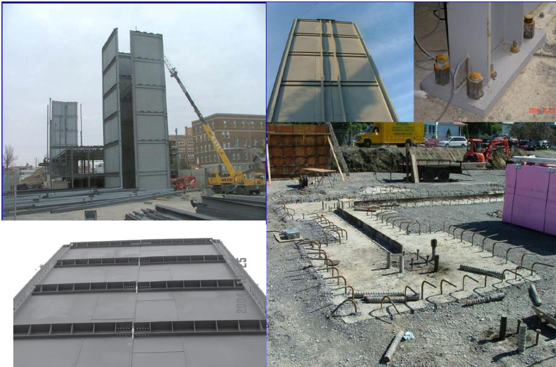
Figure 1.10 7-story ING building – mid-span splice and base connections (photo courtesy of Louis Crepeau and Jean-Benoit Ducharme, Groupe Teknika, Montreal, Canada)
