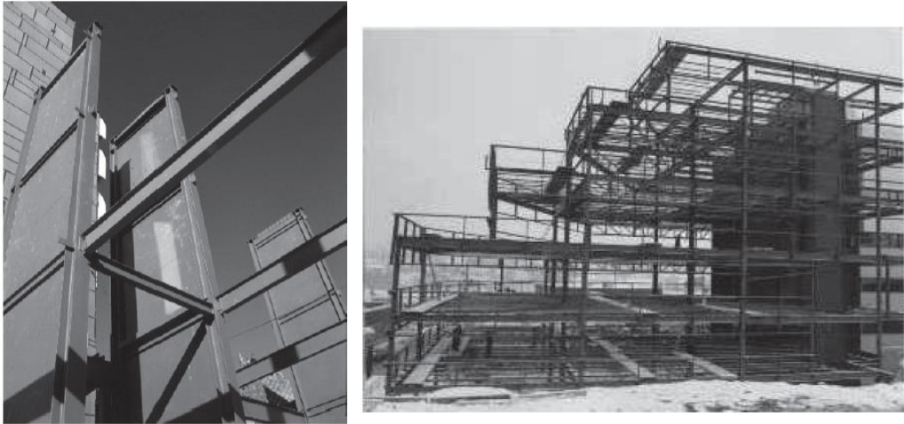
Figure 1.12 6-story Canam Manac Group headquarters expansion (photo courtesy of Richard Vincent, Canam Manac Group, St. George, Quebec, Canada)
