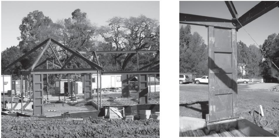
Figure 1.13 Residential building with steel plate shear wall in Atherton, California (photo courtesy of M.Eatherton, GFDS Engineers, San Francisco)
