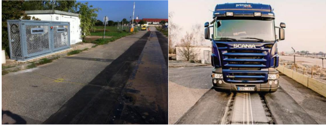
Figure 10. Electrified test track with PRIMOVE and Scania Truck [Source: Sweden Viktoria ICT]
