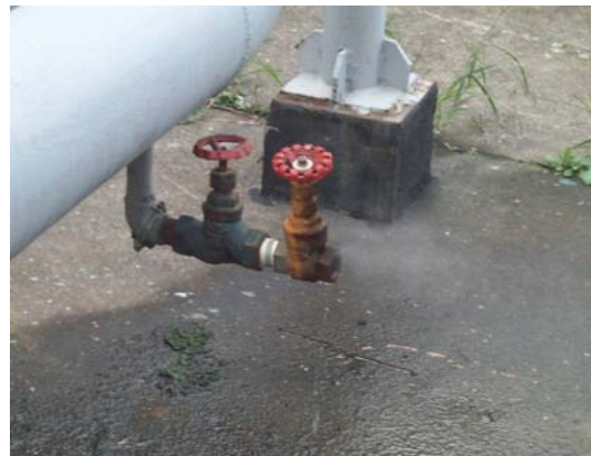
b. leaks at open valve to drain water
