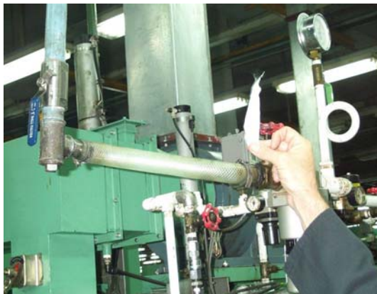
a. leaks at rubber hose connection
