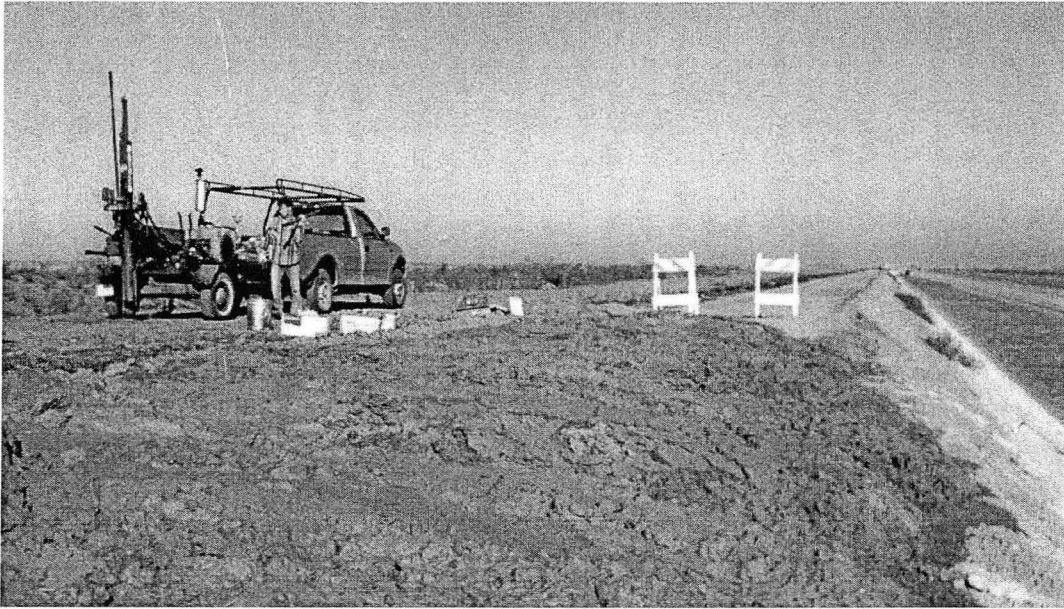
Figure C.1. Dredged SLD sediment (EP-1) drying on berm. Soil core sampling and instrument installation in progress (December 1998). View to the north.
