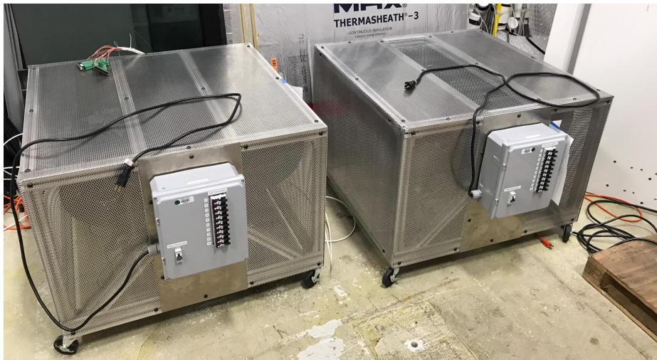
Figure 23: Load racks at the FLEXGRID.
