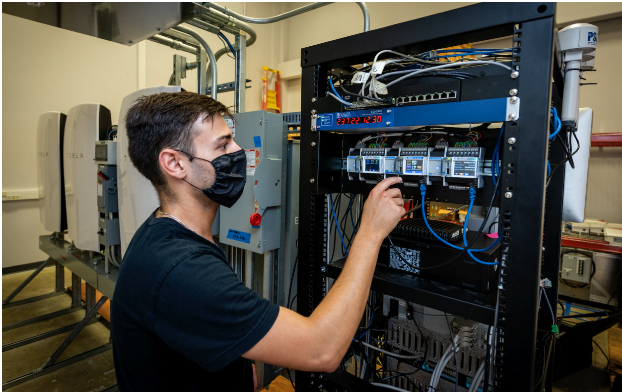
Figure 22: Maxime Baudette with micro-PMUs at the FLEXGRID. © 2010-2019 The Regents of the University of California, Lawrence Berkeley National Laboratory. Photo Credit: Thor Swift.
