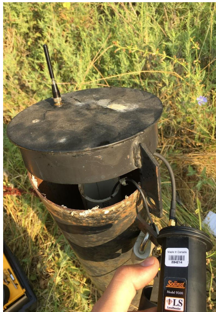
Figure A1. Installation of a telemetry unit with antenna extension in a monitoring well.
