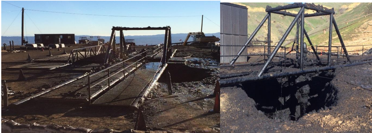
Figure 10: Vent crater caused by expulsion of top kill attempt materials.
