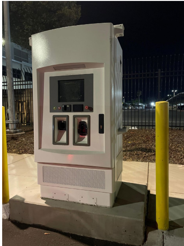
Figure 38: Damaged ZEV station from a ZEV station in British Columbia [18]
