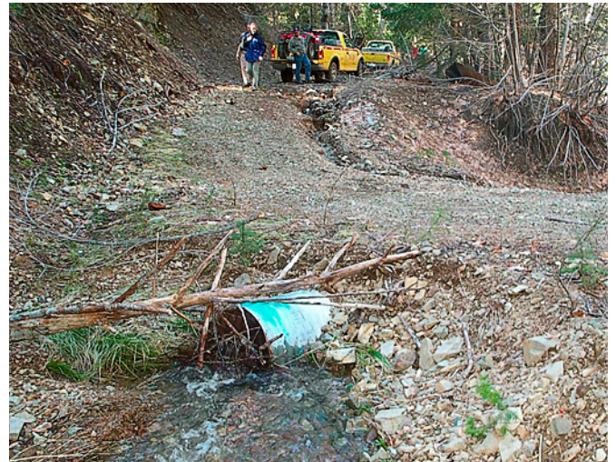
Figure 2. In this case, a culvert located uphill from the one shown plugged and diverted stream flow and sediment down the road into the stream. Photo: © Angela Wilson; used with permission.
