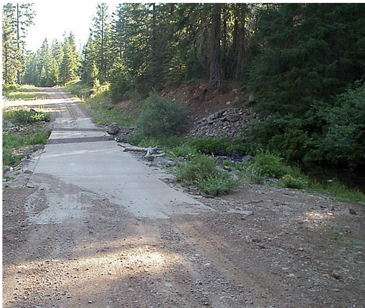
Figure 14. Concrete ford on bedrock outcrop in perennial stream. Photo: © Angela Wilson; used with permission.
