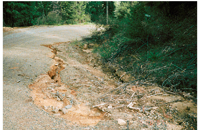
Figure 9. This ditch and road surface erosion was caused by inadequate spacing of ditch relief culverts. Photo: Susie Kocher.
