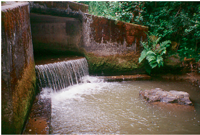
Figure 15. This box culvert will not permit fish passage because it is too high above the stream (excessive jump height for migrating fish) and the outlet velocity is too high (exceeds swimming ability of migrating fish). Any new culvert on a stream that supports fish must allow passage; many deficient culverts are being replaced. Photo: Richard Harris.
