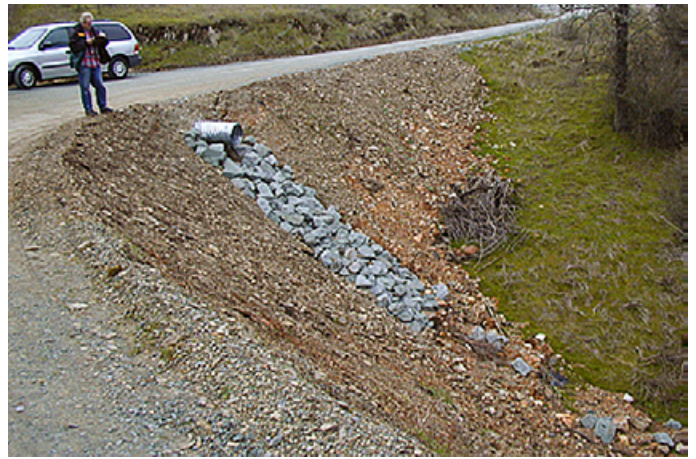
Figure 16. Rock has been installed at the outlet of this newly installed cross drain to prevent slope erosion or gullying. Photo: Richard Harris.
