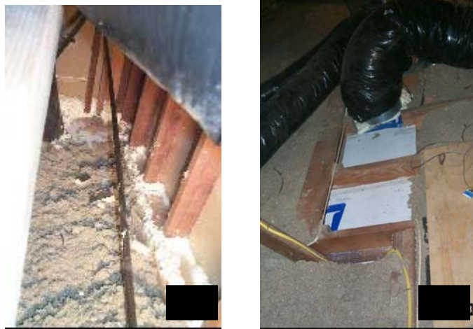
Figure 3. Sealing cavities connecting the house to the attic. Foam was used for sealing small holes and cracks at building component intersections (left). Duct board insulation was used to block off large open areas (right)
