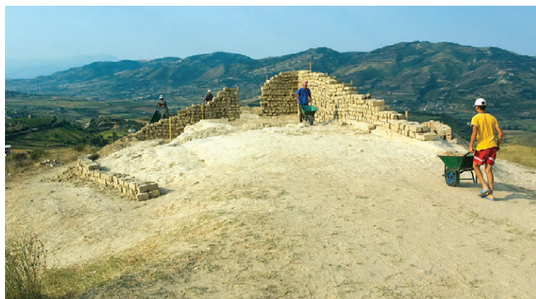
FIGURE 22.11 Mud bricks as built into a wall replicating the baulks, with openings to allow backfilling, at the end of the 2007 season (photo John Papadopoulos)
