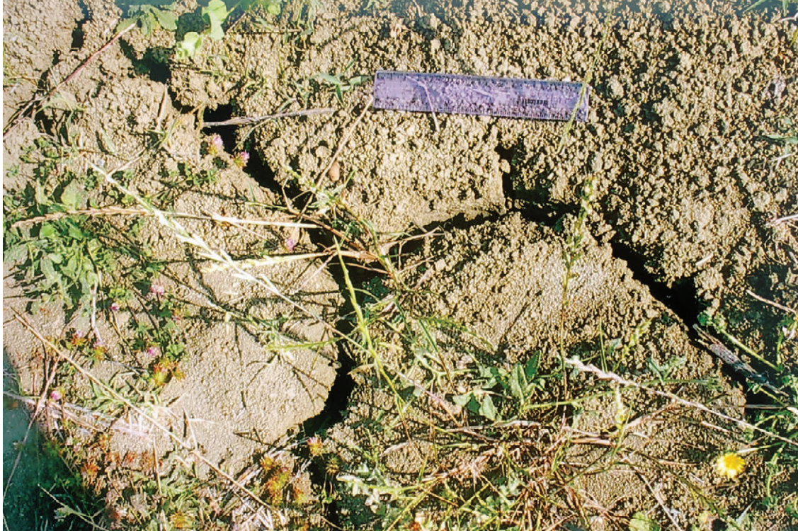
FIGURE 16.21 Cracks occurring in the shale soil during dry season. Ruler is 15 cm in length.
