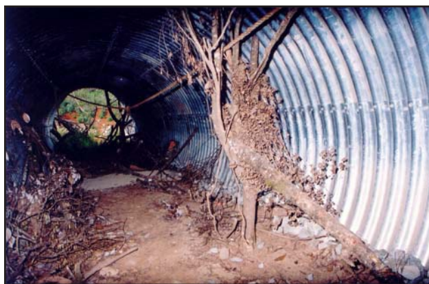
Figure 2. Faunal underpass showing furniture, including escape pole (vertical tree branch), sand bed, attractive habitat at exit, soil, litter, rocks and logs to simulate rainforest floor conditions.
