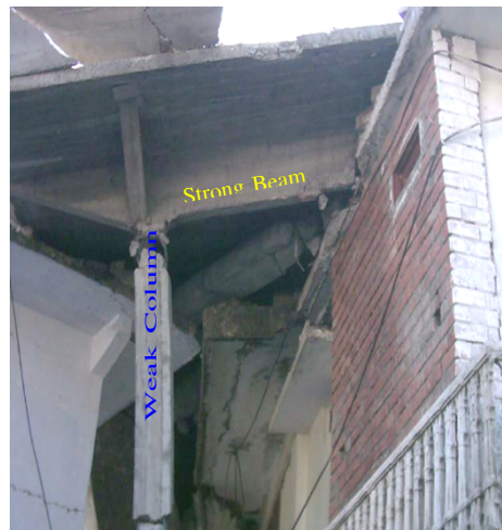
Figure (2): Weak-Column Strong-Beam Failure (2005 Kashmir Earthquake)
