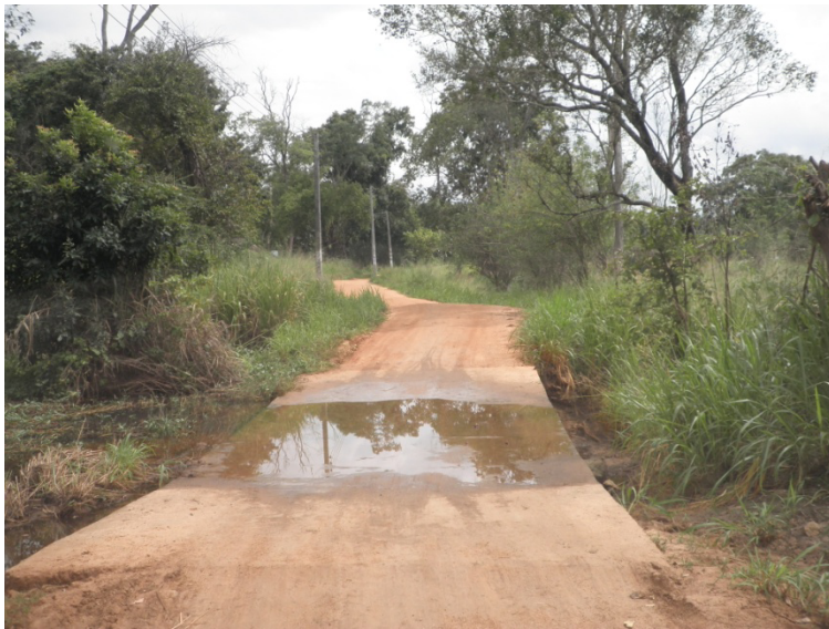
Figure 2: Poor road conditions
