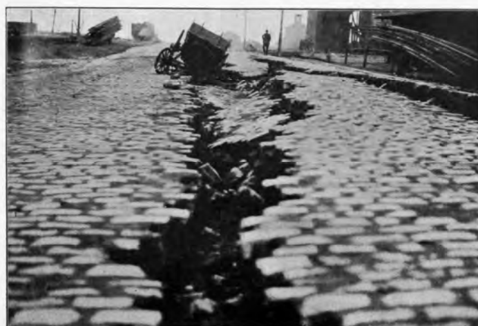
EFFECT OF THE EARTHQUAKE ON EAST STREET.
