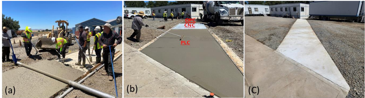
306 307 Figure 5. Slab construction (a) Rolling screed consolidation of OPC concrete (b) Trowel 308 finishing of PLC section (c) Test sections photograph after few days of casting
