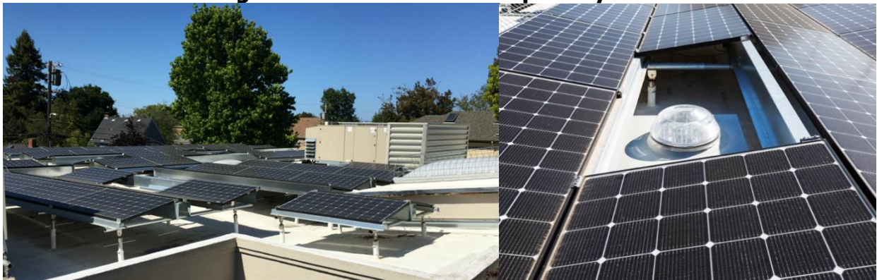
Figure 13: Installed Rooftop PV System
