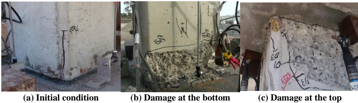
Figure 3.46 Damage propagation in column C3
