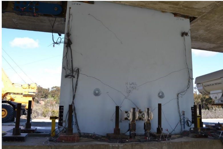
Figure 3.37 North wall damage during Phase I
