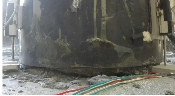
(b) South column interface, South face, \Delta=-4.5\%
