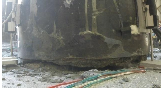
(b) South column interface, South face, \Delta=-7.5\%
