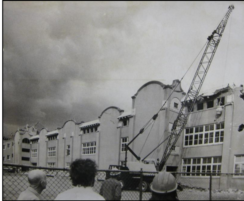
Image 14: “The last gasp for old Washington. The crash of demolition equipment resounded in the older residential part of Sacramento today as wrecking crews began tearing down the 59-year-old Washington Elementary School at 1716 E. Street. Sacramento City voters sounded the death knell for the old school last November when they approved a measure which authorizes the Sacramento City Unified School District to float up to $5.6 million ‘for the repair, reconstruction or replacement’ of certain schools which failed to meet the earthquake resistance standards of the California Field Act.” Sacramento, CA. (Courtesy of Center for Sacramento History, The Sacramento Bee Collection. 4-26-1975.)
