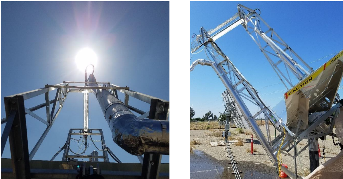
Figure 5.52 – Hybrid HCE On-Sun during May 17 th optical efficiency tests using water.
