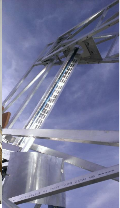
Condensation still present
