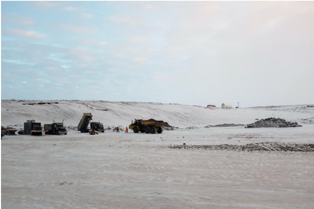
Figure 3-3. Work going on at a gravel pit off the ITH. Source: Author, April 2017.
