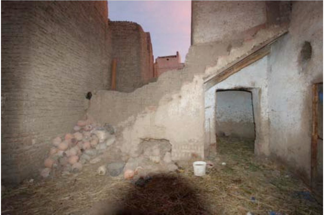
Figure 6. In Al-Biirat: Floating brick stairs supported by halved palm trunk (far side) and a single train-track rail (photograph by author).
