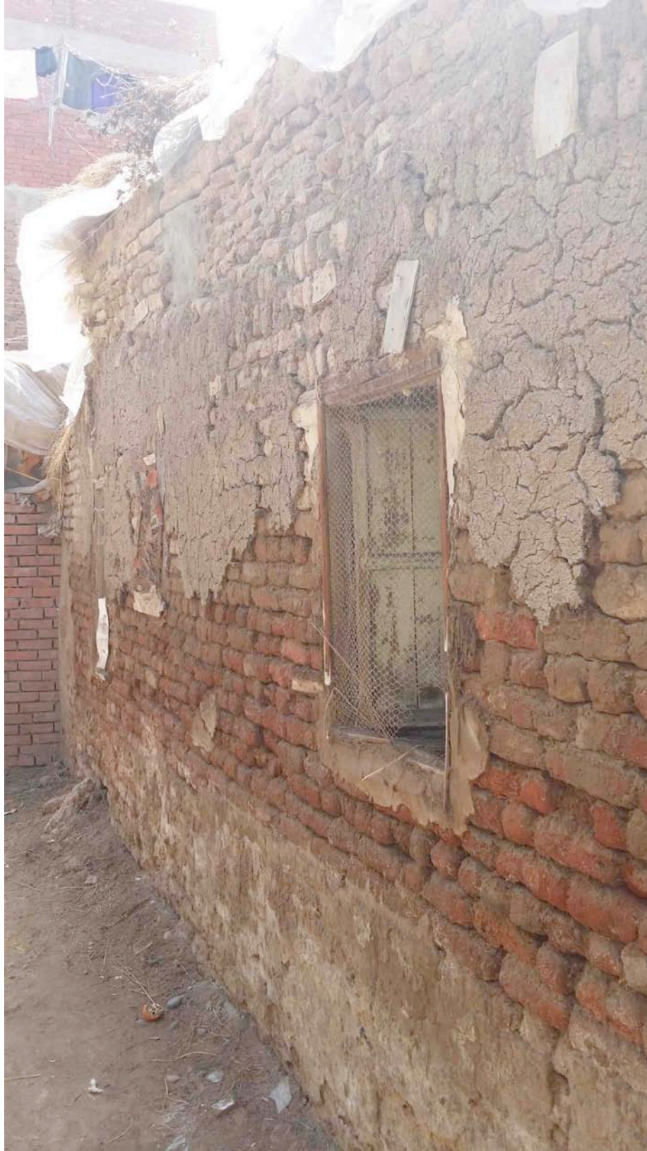
Figure 47. House Four: The house is constructed of plastered red brick (photograph by author).
