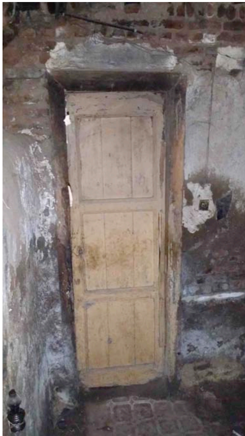
Figure 50. House Four: The interior walls exhibit the consequences of moisture and salts (photograph by author).
