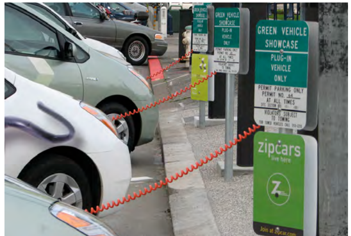
ZipCar Charging Station - San Francisco , For profit private vehicle rental companies oriented toward local residential use, such as Zipcar, Flexcar, and Car2Go.
