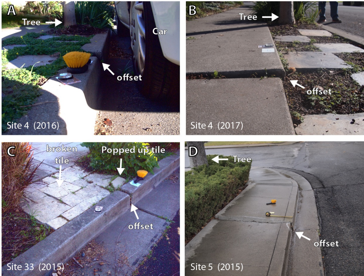
Figure 3.12: Field photos of sites 4, 5, and 33 which show nearby trees that can influence curb movement (A and D), parked cars that obstruct the view of taking photos from different vantage points (A). Also observations of offset pathways adjacent to the offset curb (B), and broken, popped up tiles in between a pathway and offset curb (C).
