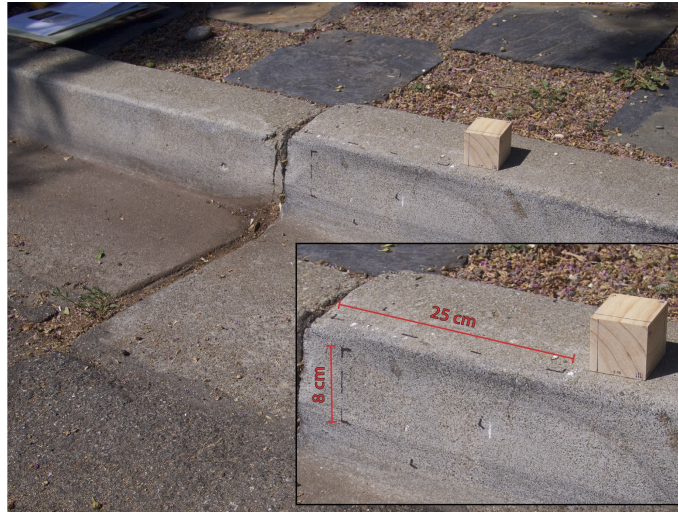
Figure 3.30: Site 4 in 2017 showing black permanent marker markings on the vertical and horizontal planes of the curb.
