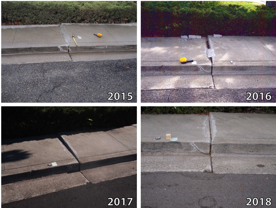
Figure 3.4: Variations in curb photo setup and weather conditions. In 2015 and 2016 we used a tape measure, compass, and brush. In 2017 and 2018 we used a compass and 5 cm block. The overcast weather conditions in 2015 and 2018 show more defined details where as the sunny conditions in 2016 and 2017 which introduces unwanted shadows.
