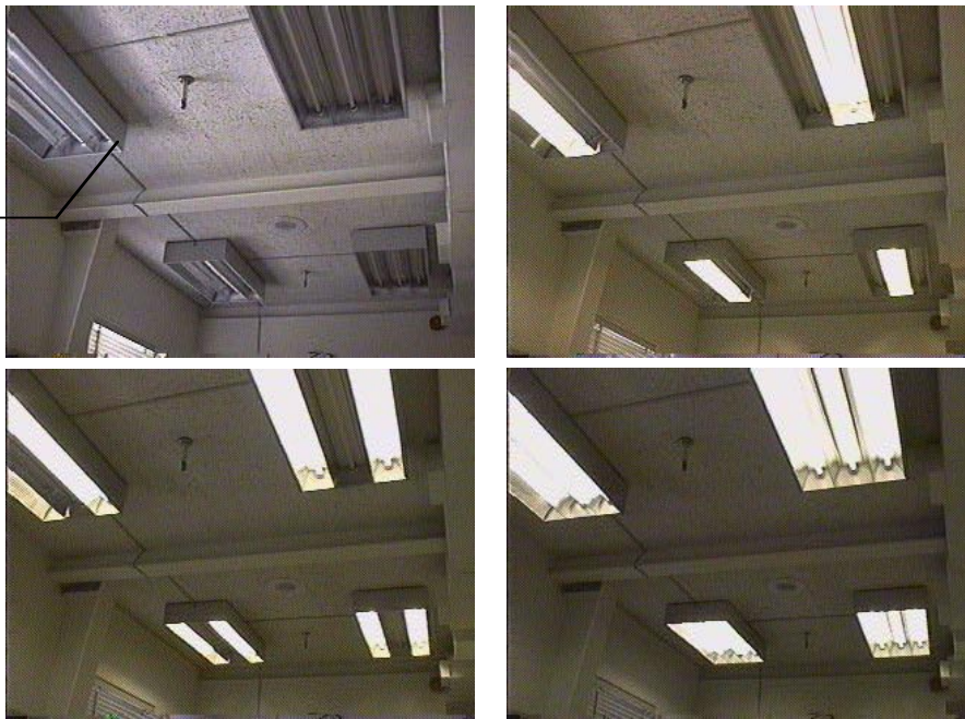
Figure 5. Images of the ceiling lights in office at LBNL Building 46 where the IBECS network interfaces were first tested. The upper left image shows the lights with both wall switches in the OFF position. The location of the installed low-voltage wire raceway is shown in the callout. The upper right image shows the lights with the in-board switch ON and the outboard switch OFF. The lower left image shows the lights with the outboard switch ON and the inboard switch OFF. The lower right image shows the lights with both switches in the ON position.
