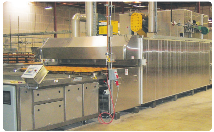
The tunnel oven at Alvarado Street’s bakery in Petaluma represents a major investment in the new facility.
