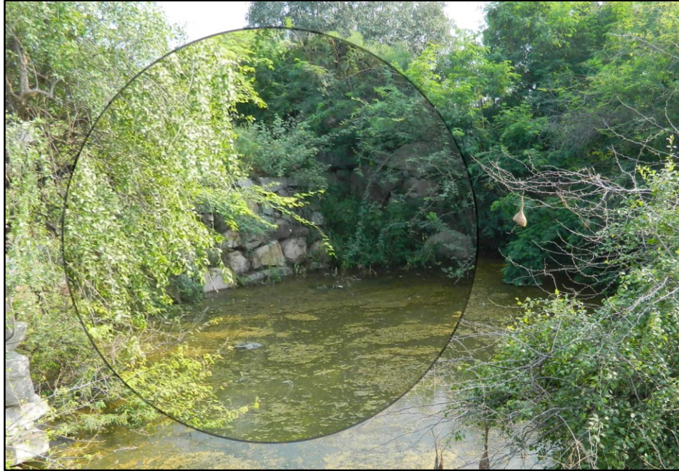
Fig. 5-19: Hampayyanna Bavi (G15) masonry (magnified inside the circle), overgrown with vegetation. This is located to the north-west of the village.
