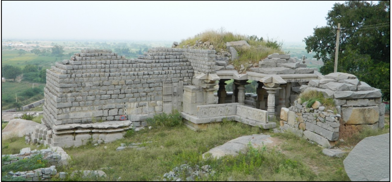
Fig. 5-53: Staggered square plan of the shrine at Suguresvara temple, looking NE. Only part of the original architecture around the shrine is preserved, but one can spot kuta-stambha aedicular component being used here.
