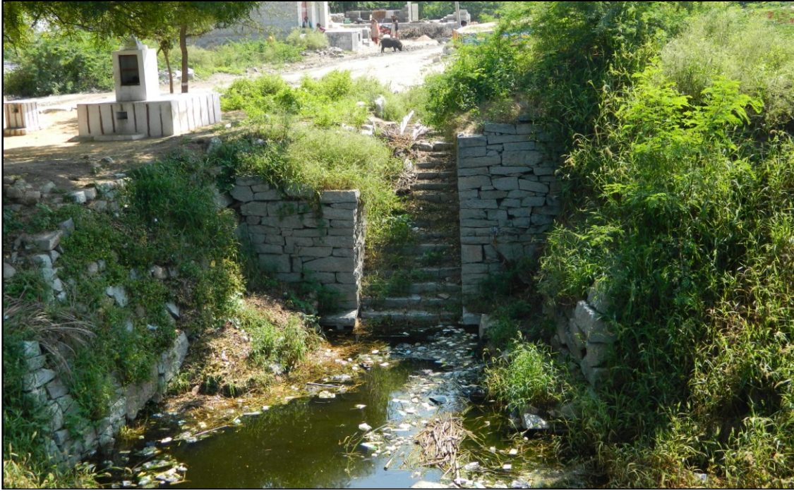
Fig. 5-32: Southern masonry and stairs of the well next to Balanjaneya temple (G1)
