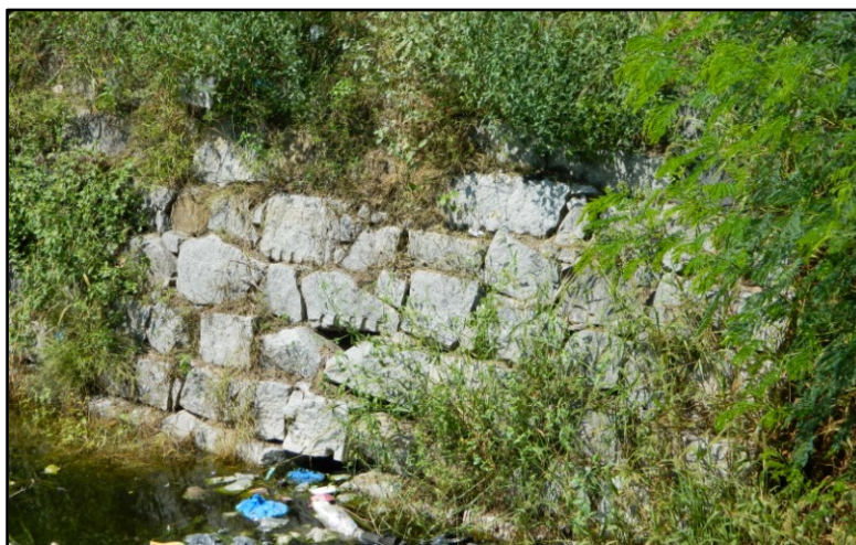
Fig. 5-20: Well at G1, in the complex of Balanjaneya temple, next to the northern boundary and entrance of the Gabbur village.
