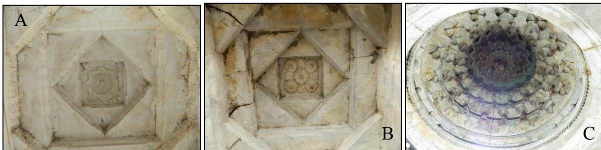
Fig. 5-48: Ceiling constructions at Mel Sankara temple (A and B) at G28 and Venkateshvara temple (C) at G5.
