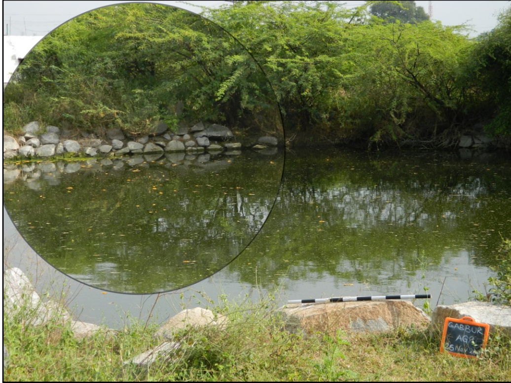
Fig. 5-17: Masonry of a well in the fields South of Gabbur village (G77)
