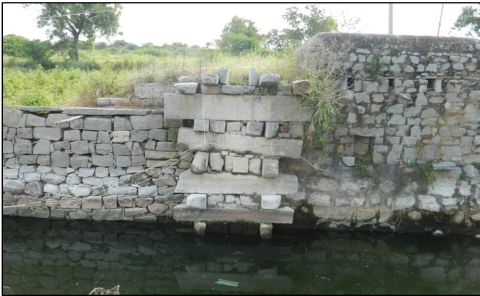
Fig. 5-40: Taiamma Bavi (G86), new masonry repair work visible along the southern edge. A broken pitha and water channel were found next to this well.
