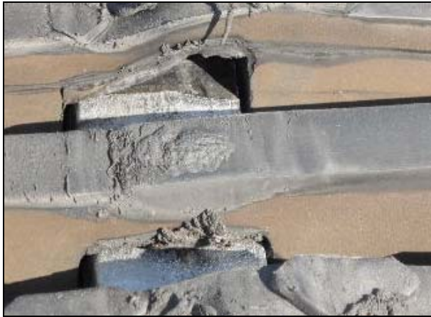
Figure 4.66: Phase 3.3: Damage to steel rib of Trelleborg unit.
