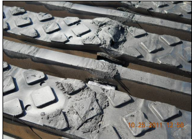
Figure 4.67: Phase 3.3: Deformation and shoving of rubber on Trelleborg unit.
