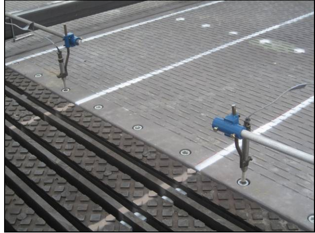
Figure 3.9: LVDTs on Trelleborg unit. (Instruments #8 and #9)
